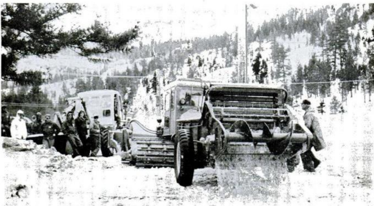
Pulvi-Mixer, below, grinds sawdust into the top six inches of snow. The surface is allowed to set for about 40 hours before testing. Test pad successfully bears a load of 200 vehicular tons at one time
