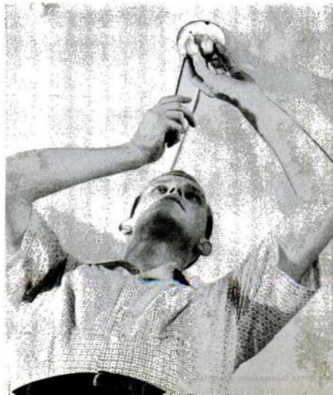
Installation of detector unit is done with screws. Wire leading to central panel (left) is stapled into place
