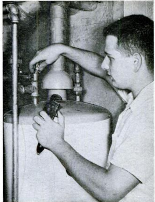
8 Safety valve at top of heater tank is disassembled so that destroyed fusible plug can be replaced
