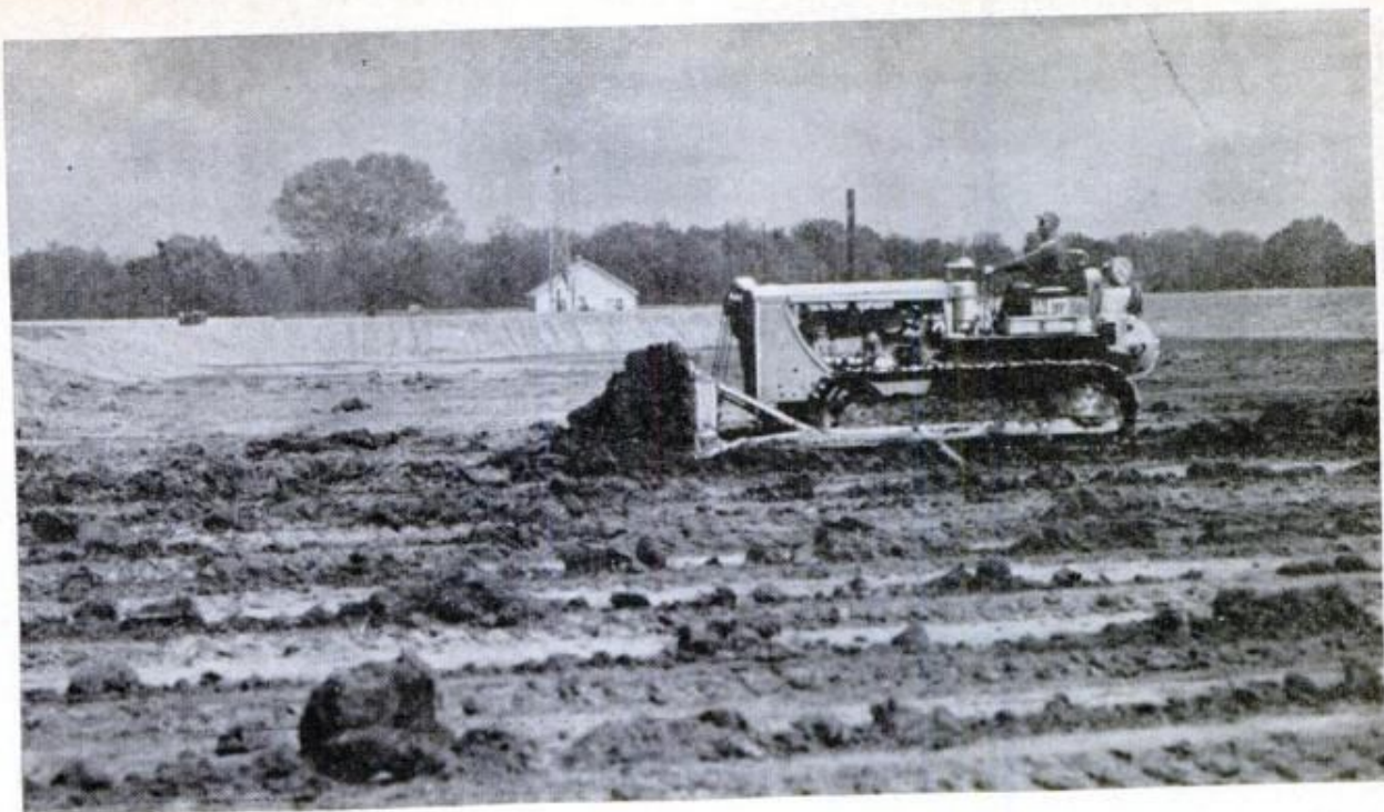
Caterpillar tractor operator raises up dikes to hold three feet of pond water
