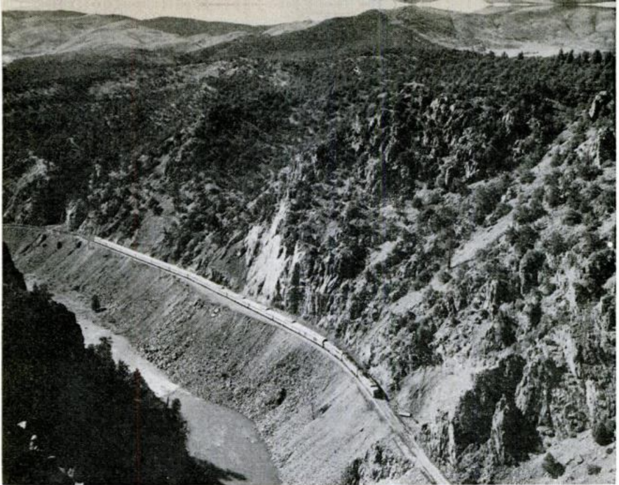
As soon as the rubble stopped falling, two big shovels and dozens of men went to work pitching tons of pulverized granite over the side into the canyon. As they worked, track-laying crews followed at their heels installing the temporary tracks. Within one hour the eastbound California Zephyr, above, passed safely over the spot where only a freshly scarred rock outcrop marked the location of the old Gore Canyon tunnel
