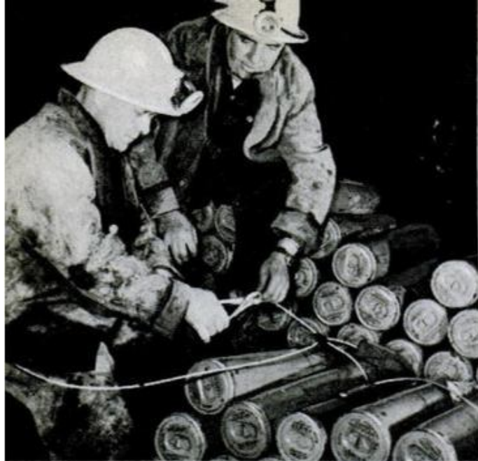
Deep inside Ripple Rock, DuPont engineers crimp detonating cord to canisters of Nitramex blasting agent. The cord detonates at the amazing rate of 20,000 feet per second, allowing instantaneous detonation of widely separated charges
