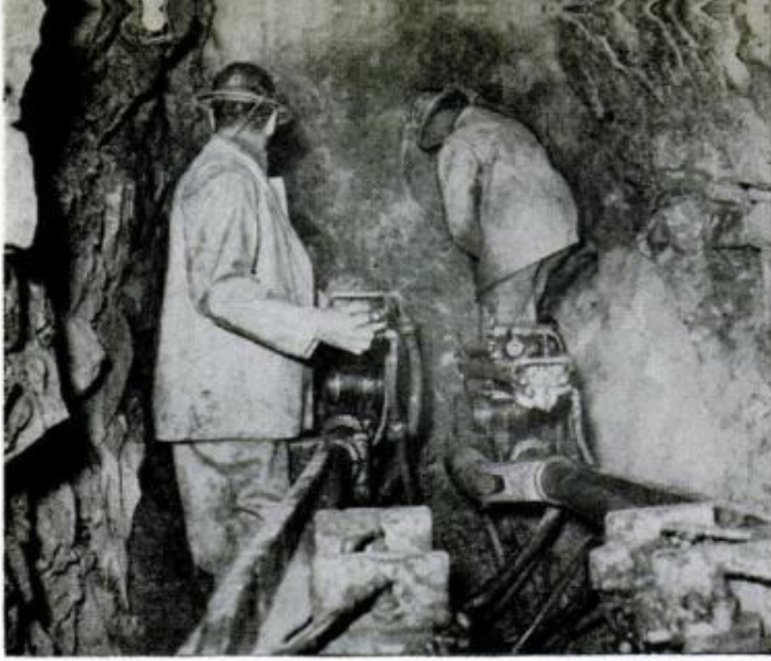
Workmen digging part of the 500-foot labyrinth of coyote tunnels used in the famous Promontory Point blast in Utah, which yielded three million tons of fill rock for a causeway across the Great Salt Lake. The blast is called by explosives experts "the riskiest coyote shot ever fired"
