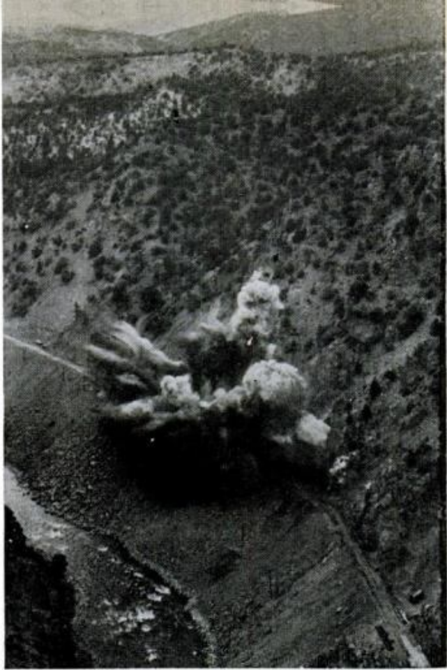
Immediately after the train had passed, Atlas experts fired a huge single blast calculated to blow the entire granite outcrop out into the canyon. 25,000 tons of rock had to be removed without damaging the busy roadbed beyond immediate temporary repair
