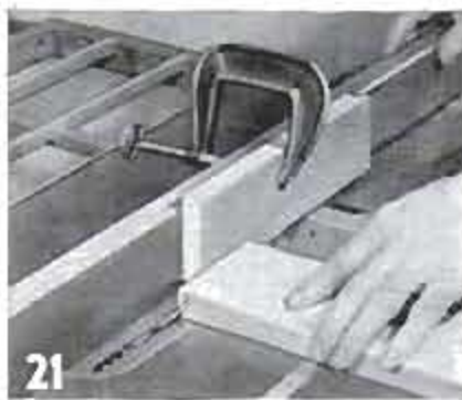
21 Tilt blade to 45 deg. and miter corners on all ends marked B
