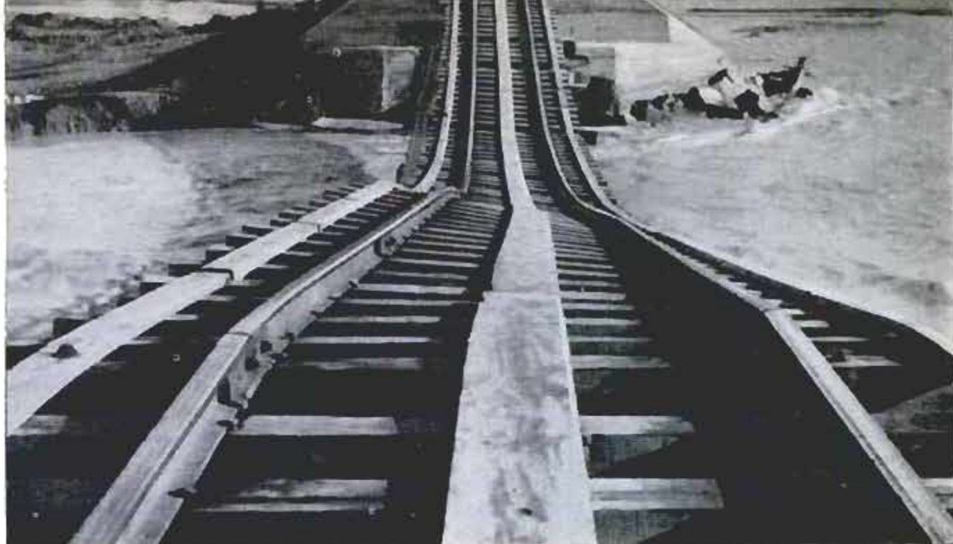
Rails are left hanging in air after a flood washed out bridge supports. Floods present a constant threat
