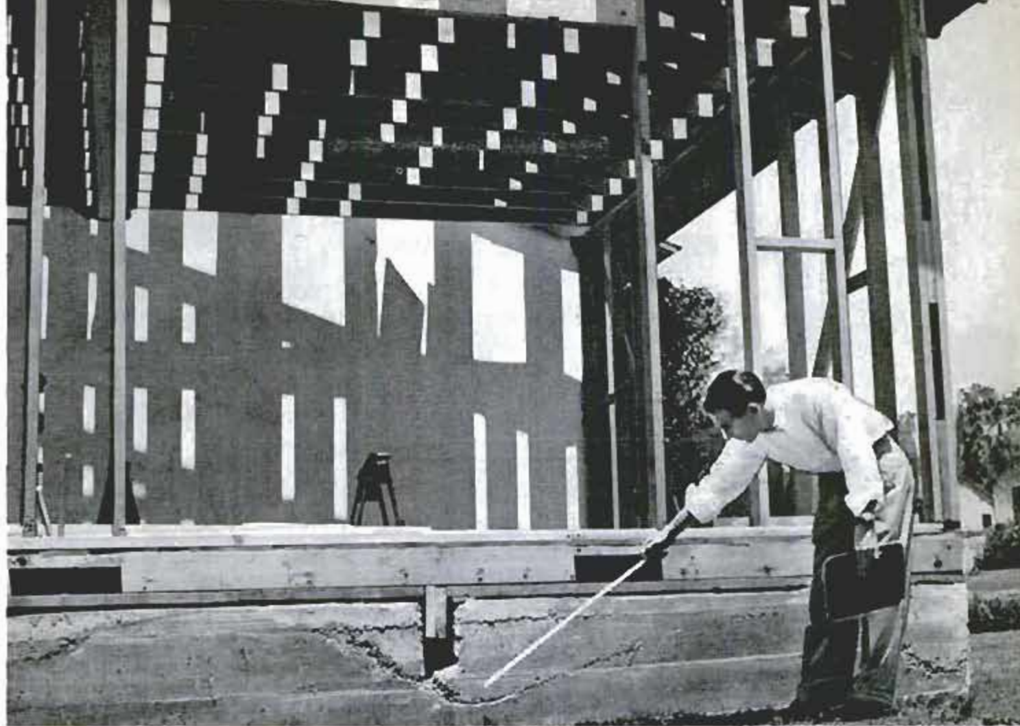
Inspector notes cold joint in concrete foundation. Fault occurs when too much time elapses between pours
