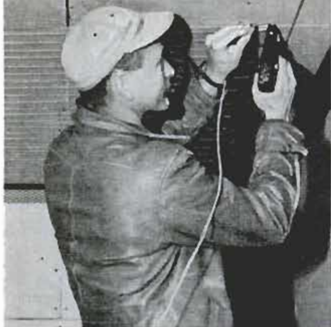
In the hidden ceiling-coil system, resistance coils are stapled in place on an unfinished ceiling
