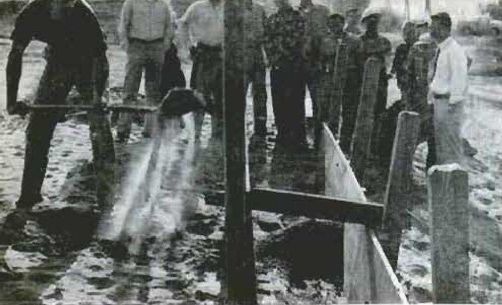
Students watch demonstration of how to fill mud box. Box is two parallel wooden walls held together with cross beams and stakes. Mud boxes hold back flood waters and take place of sand bags when solid fill is scarce
