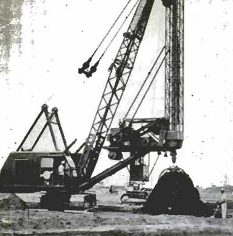
Enormous earth drill is used to bore holes for concrete piles that support tall steel-frame buildings
