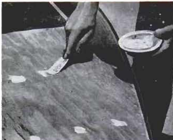
1. Above, after paint is removed from deck, voids and depressions are filled with non-oil-base putty
