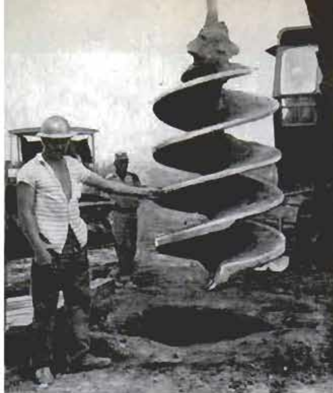
Drill has penetrated 120 feet to reach compact earth. Untrained Brazilians have become top-notch workers
