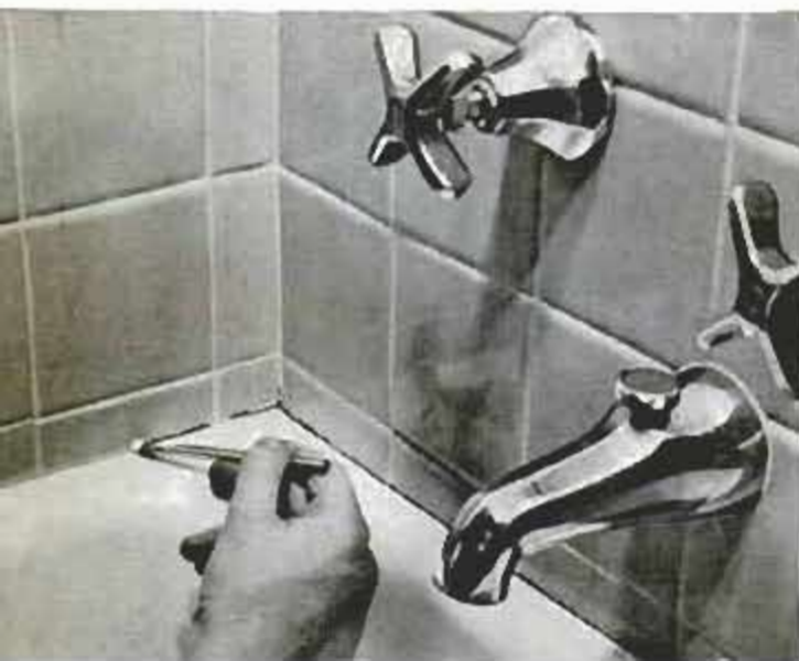
Hysol, another epoxy brand, was used by homeowner in calking edge of bathtub, common place for leaks
