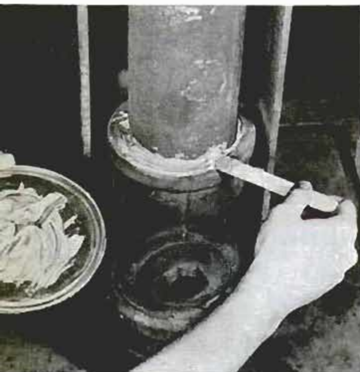
One-to-one mixture of epoxy resin elements from two tubes was used in making repairs on leaky pipe
