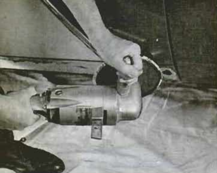
In employing a plastic metal like Liquid Iron for auto body repairs, area to be filled is first sanded
