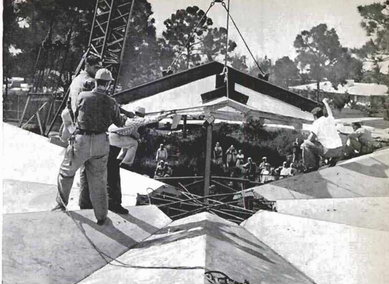
Last section of the "piecrust" roof is eased into place; open space in the center is for a big skylight
