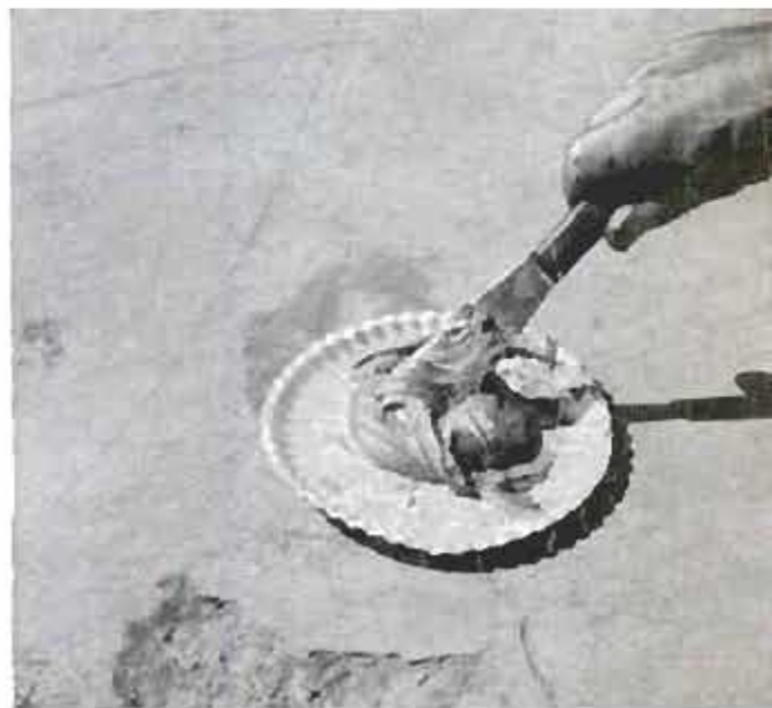
Another job for the new glues is patching concrete. Here a batch of Plastic Mastic is mixed
