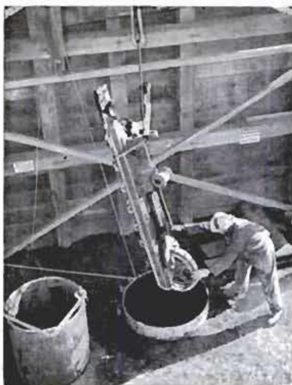
Part of a 3½-ton tractor starts trip through 42-inch-wide shaft to deep gas-storage cave
