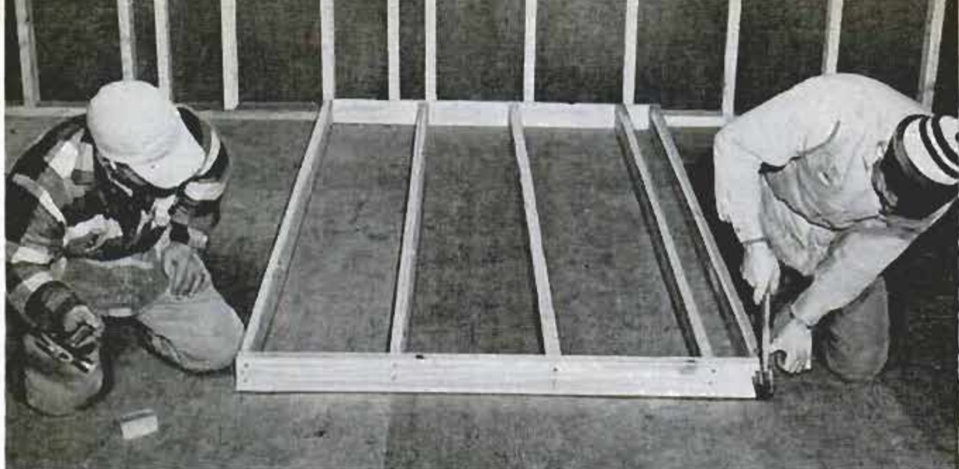
Partitions are built as panels on floor, using group of studs cut to identical lengths in cutoff jig
