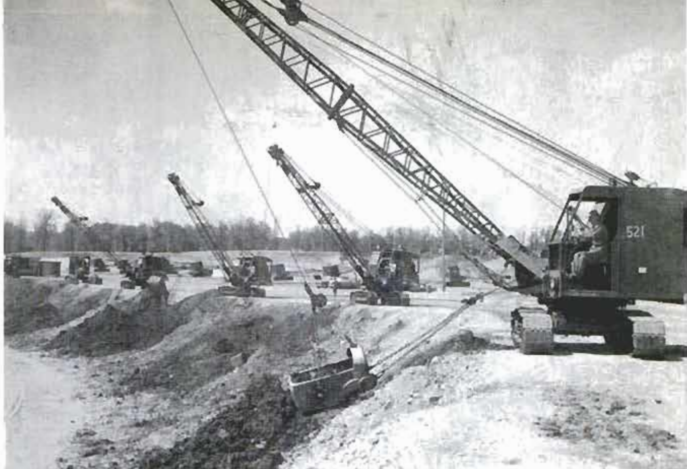
Shovel-and-dragline students get feel of their machines—probably hardest construction tool to handle
