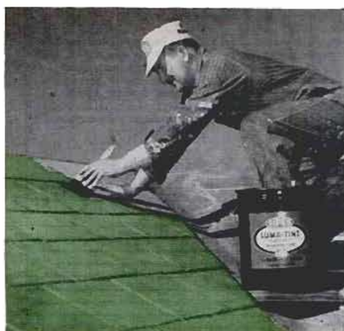
Thomas Wittas says it was an easy, one-day job to restore his roof with Luma-Tint Colored Aluminum Coating. Luma-Tint is made by James B. Sipe & Co., Pittsburgh, Pa.
