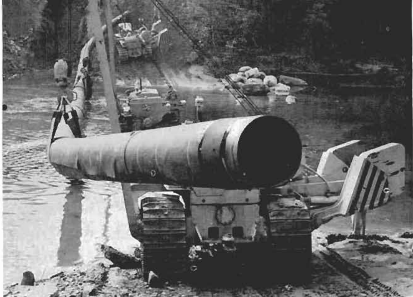
Diesel-powered tractors equipped with side booms position pipe where line crosses river in Pennsylvania
