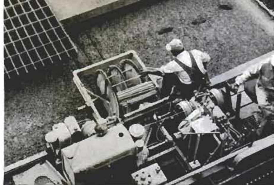
Device called a tie-in wheel places the center tie rod beneath the surface of the first layer of concrete before steel mesh is positioned
