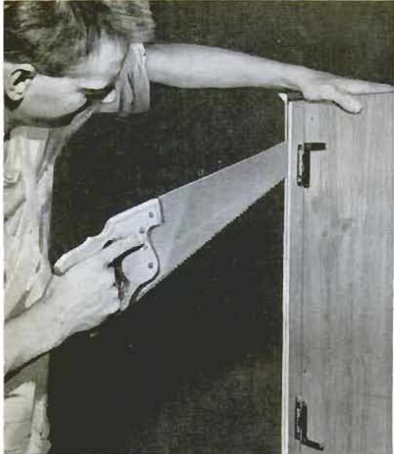
Above, cabinet corner member is cut along line marked on tape so that it fits flush against wall having irregular surface
