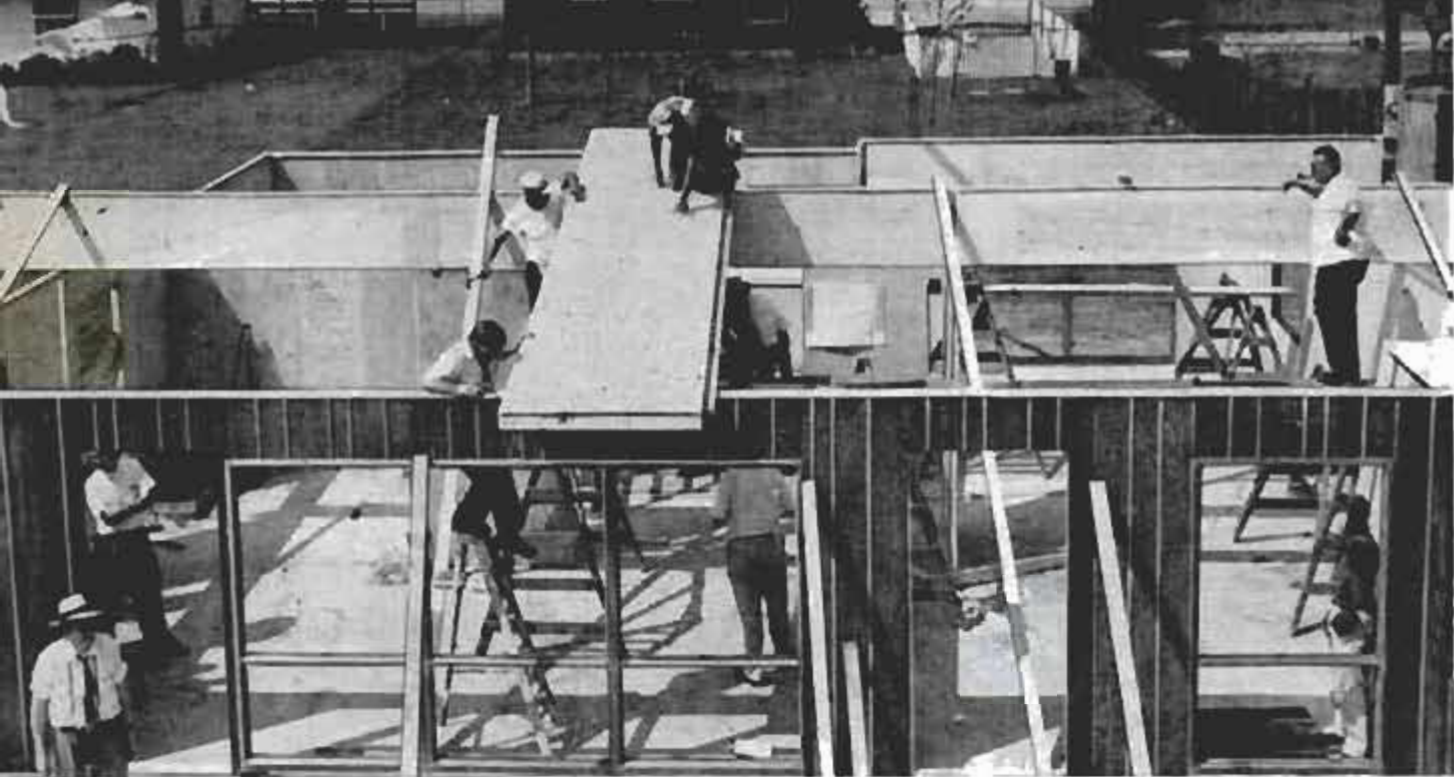
First of plastic-core roof panels is put on South Bend house, which five men erected in one working day
