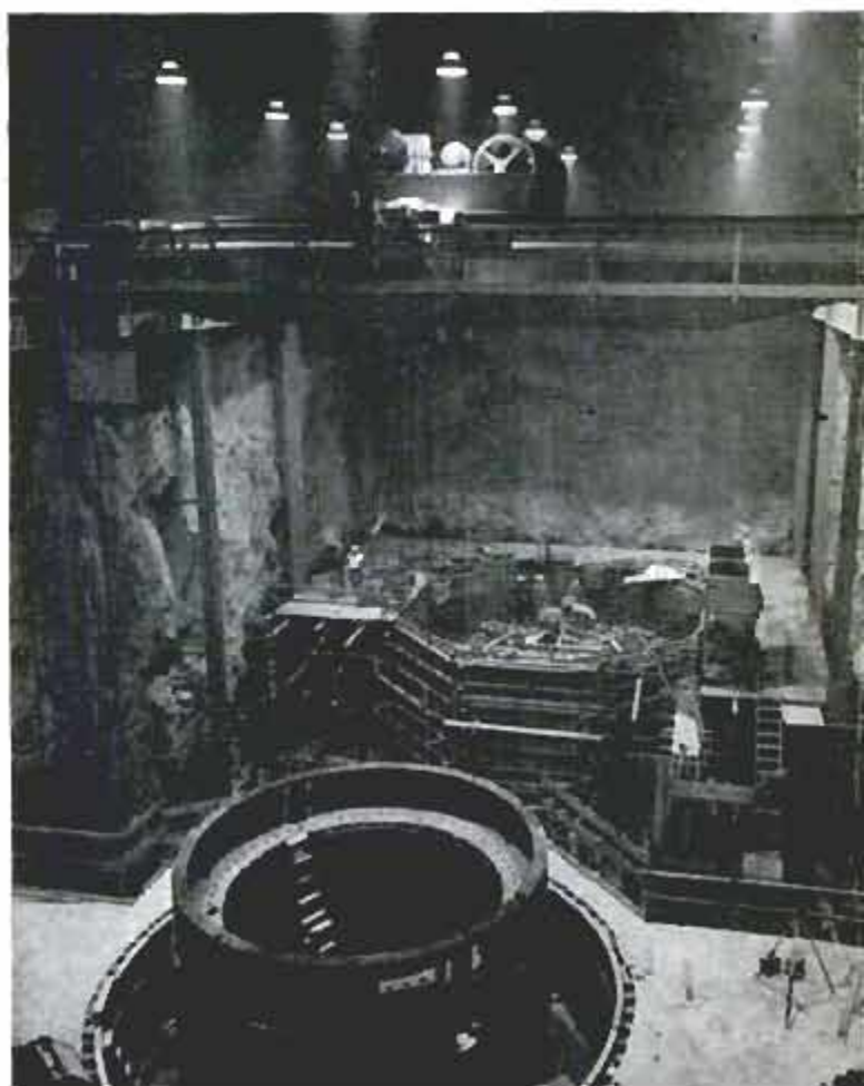
Interior view of underground powerhouse during installation of generators. Walls are solid granite
