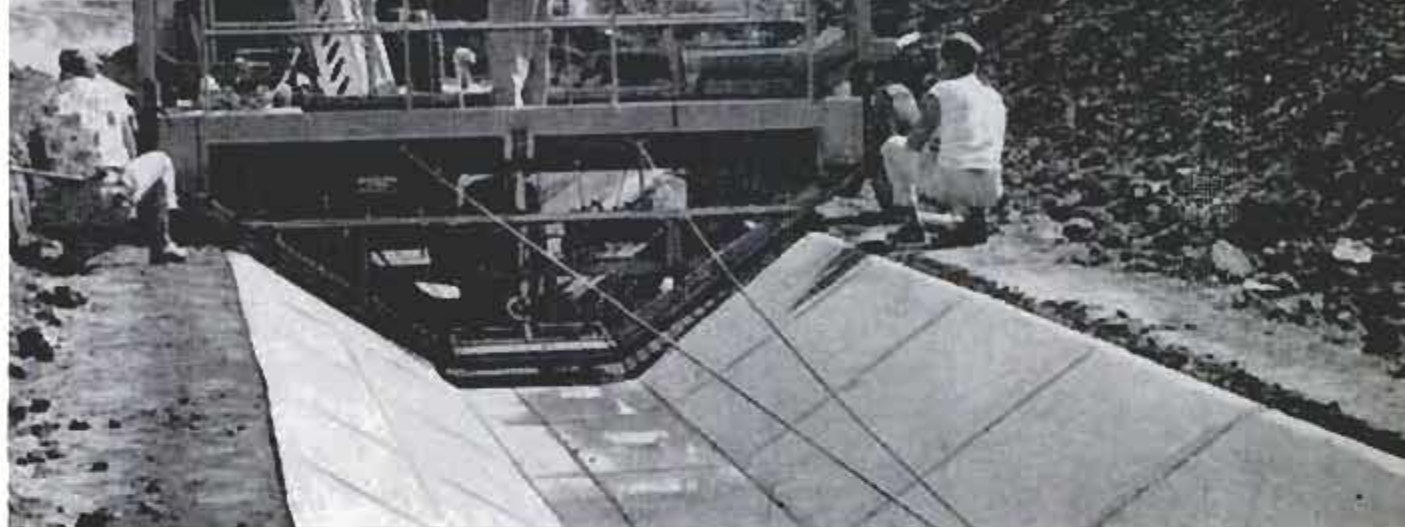
Ditch left by huge shovel can be surfaced with concrete by machine that travels behind the ditch digger
