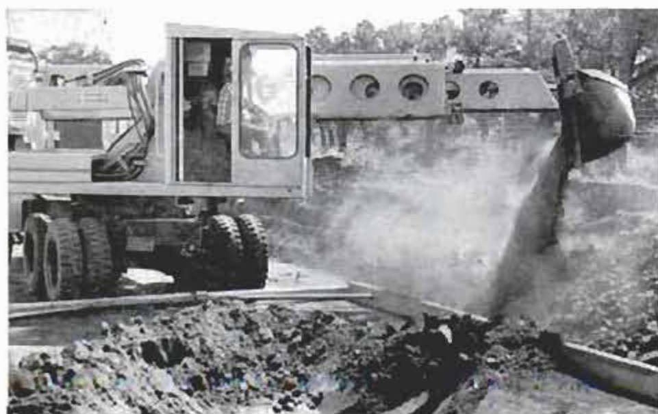
When shovel is filled, the boom is lifted and swung to one side. Shovel then is tilted and dirt is dumped beside the new ditch. When machine moves ahead, shovel is positioned for next bite
