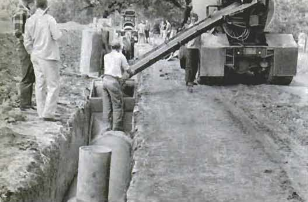
Continuous concrete pipe is produced in ditch which has curved floor. Fresh concrete runs from truck into hopper at rear of form-packing sled
