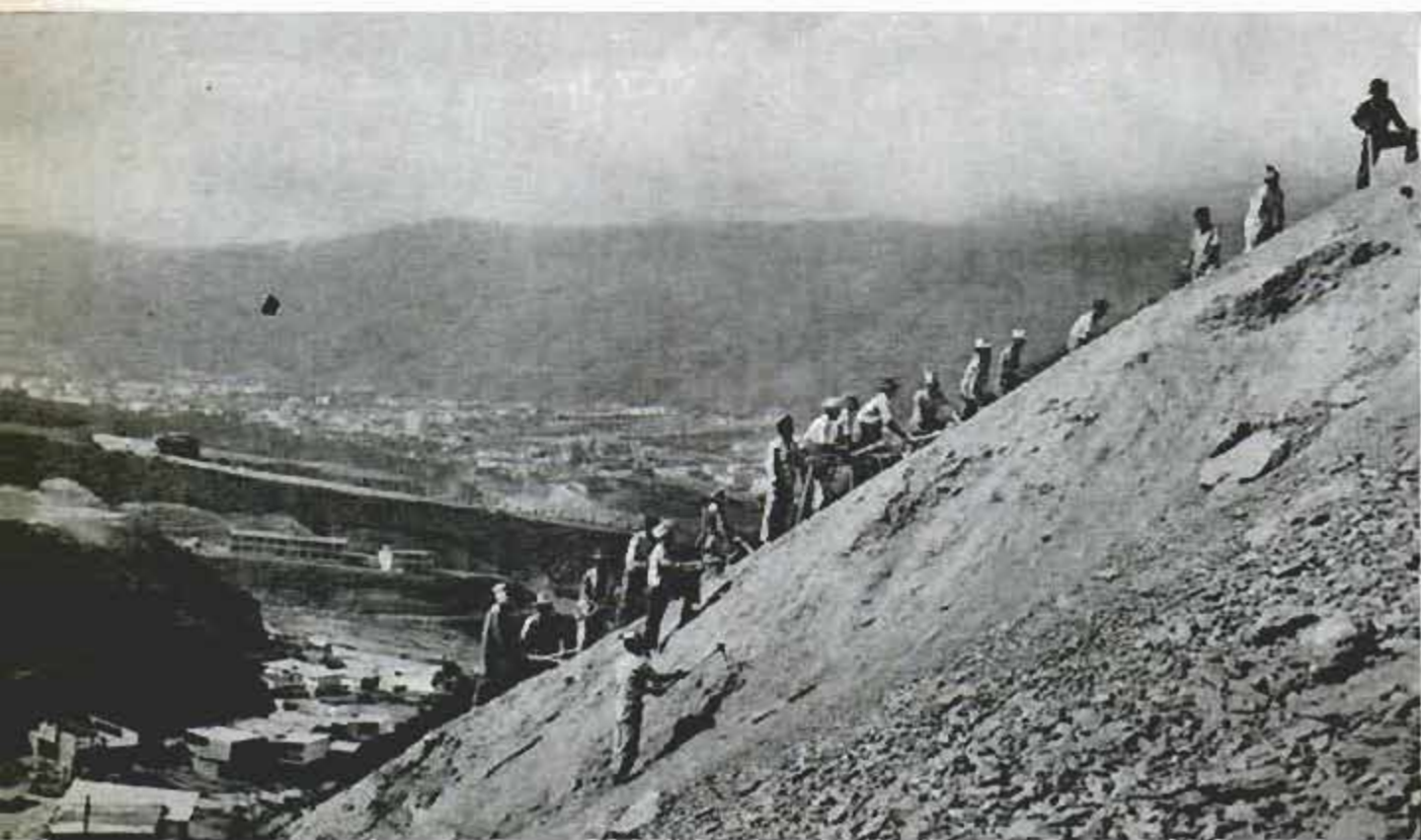
Gang of workers terraces mountainside above Caracas to prevent erosion. Grass will be planted on terraces
