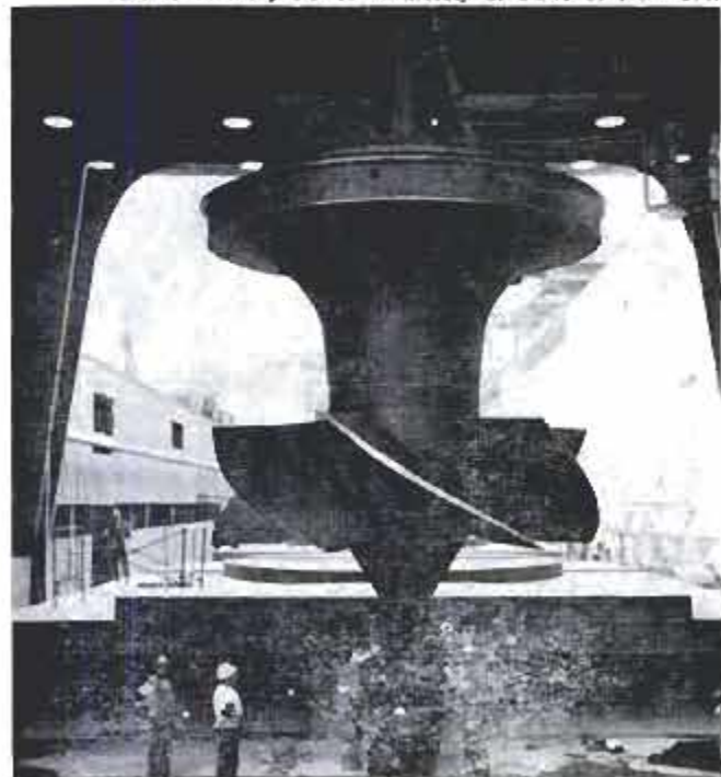
Huge turbine runner assembly for one of the dam's generators is moved into lowering position by gantry Photo courtesy Power Authority of State of New York
