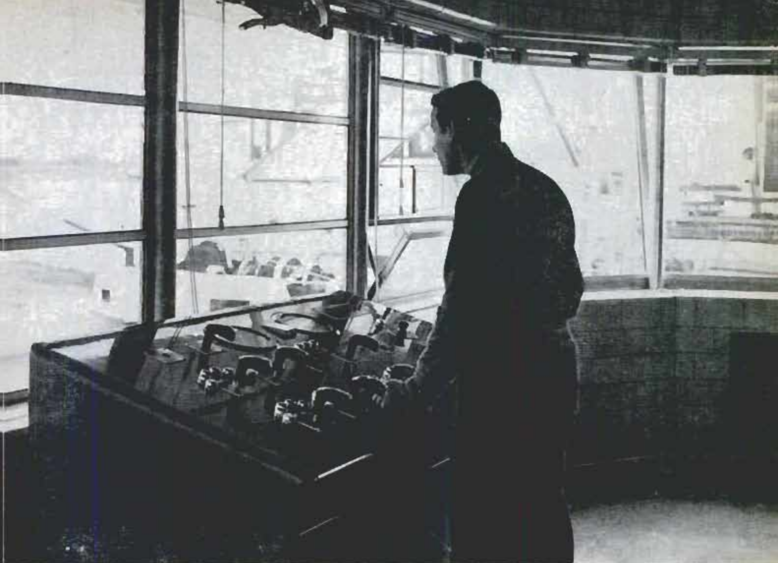
Controls for lock valves and gates are on console. Warning lights prevent operator from making mistakes
