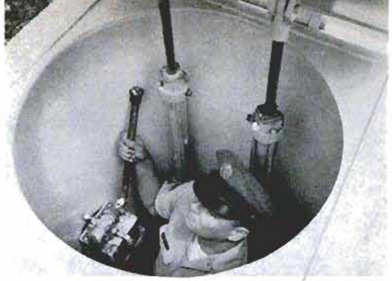
Air Force technician works manual pump to open escape hatch. An Atlas blockhouse, below, is partially beneath ground level
