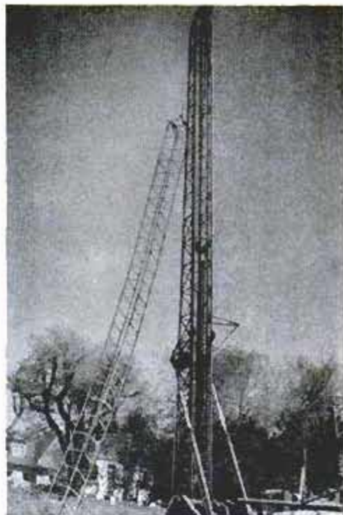
A drilling unit hoists a reinforcing assembly for dropping into the bored hole
