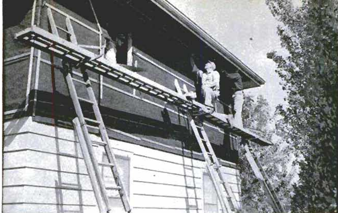
Neighbors pitch in to help Cal Schroeder with the sheathing. Big overhang helps appearance of the house
