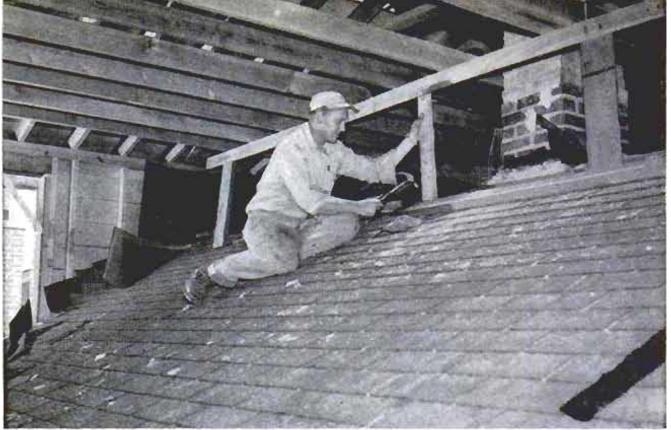
So family could continue living in home during remodeling, old roof was left in place until new one was up
