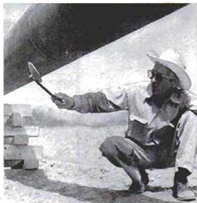
Outside rear-view mirror from car is used to inspect welding before the pipe is lowered into ditch
