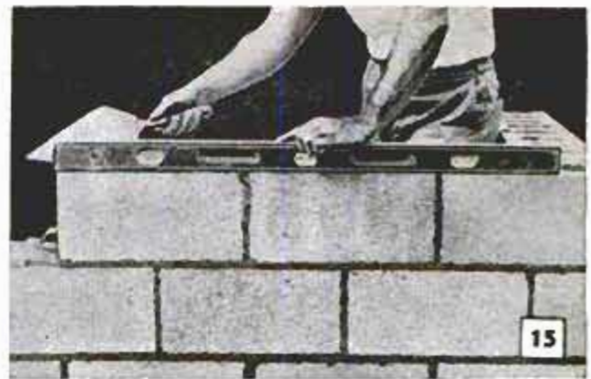
As each block is placed on mortar bed, it is leveled. For this job a long level is better than a shorter one
