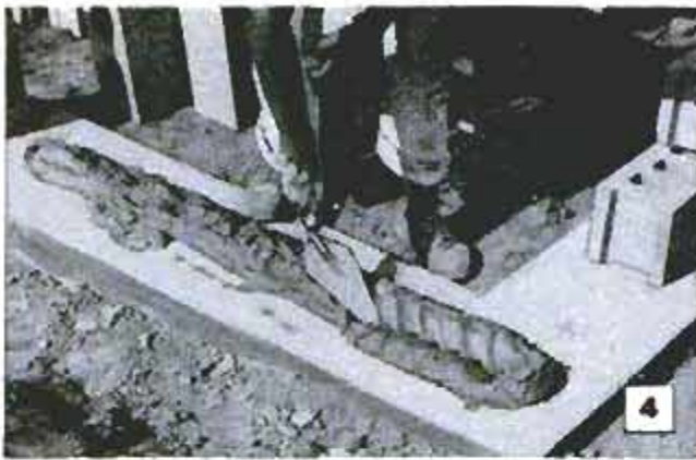
Full bed of mortar is spread on foundation to receive first course of block, assure maximum strength
