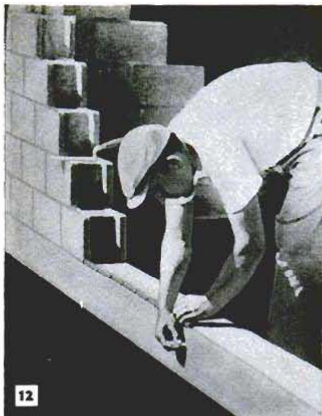
Marking off foundation, or laying out blocks without mortar, indicates required spacing of blocks or need of partial block between built-up corners
