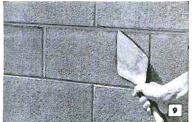
As blocks are placed, trowel is used to remove excess mortar, trowel point compacts mortar in joints
