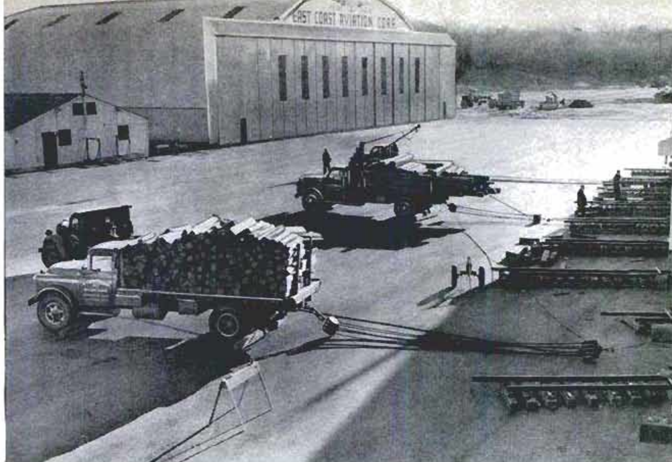
Weighted tow trucks "on the mark" ready to take up slack in block-and-tackle system and get hangar moving
