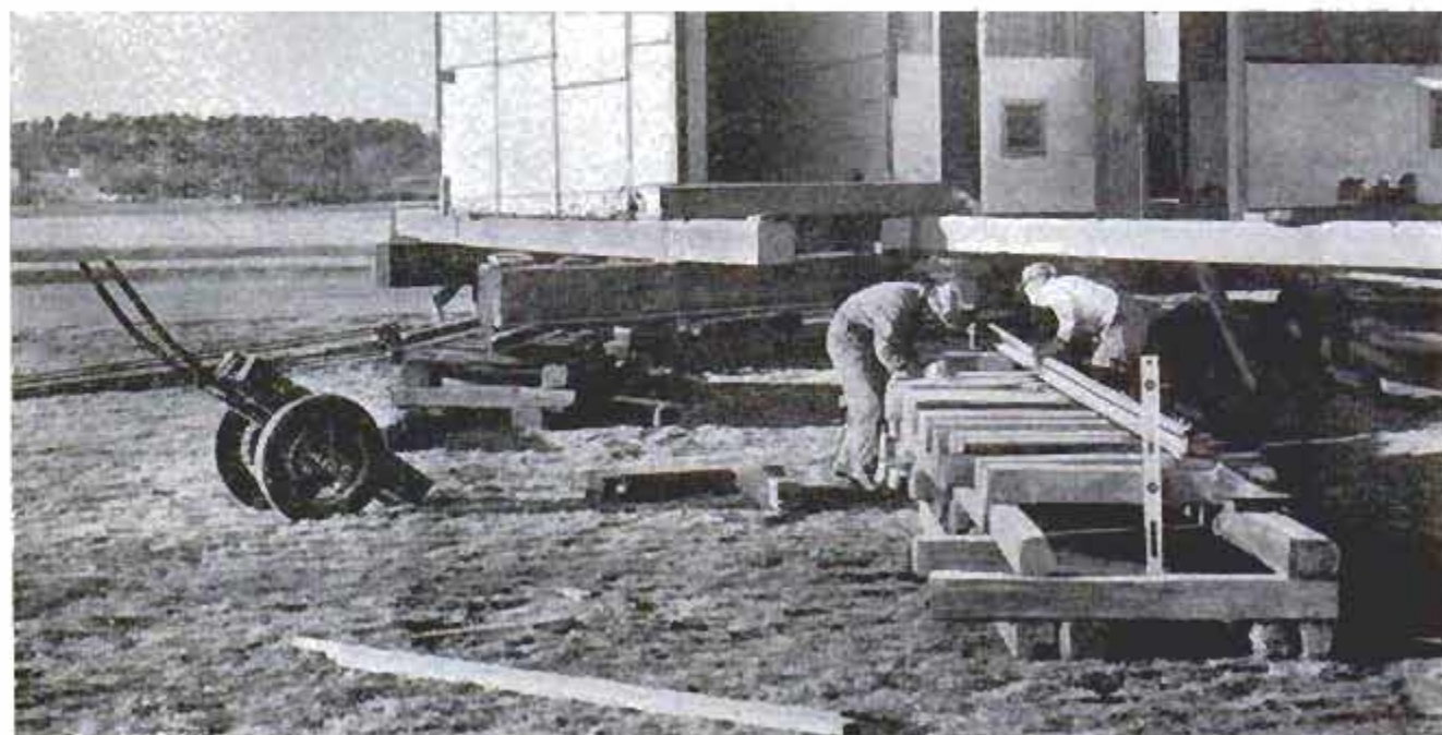
Workmen adjust track bed for moving the hangar. Timber bed must be kept level regardless of the terrain
