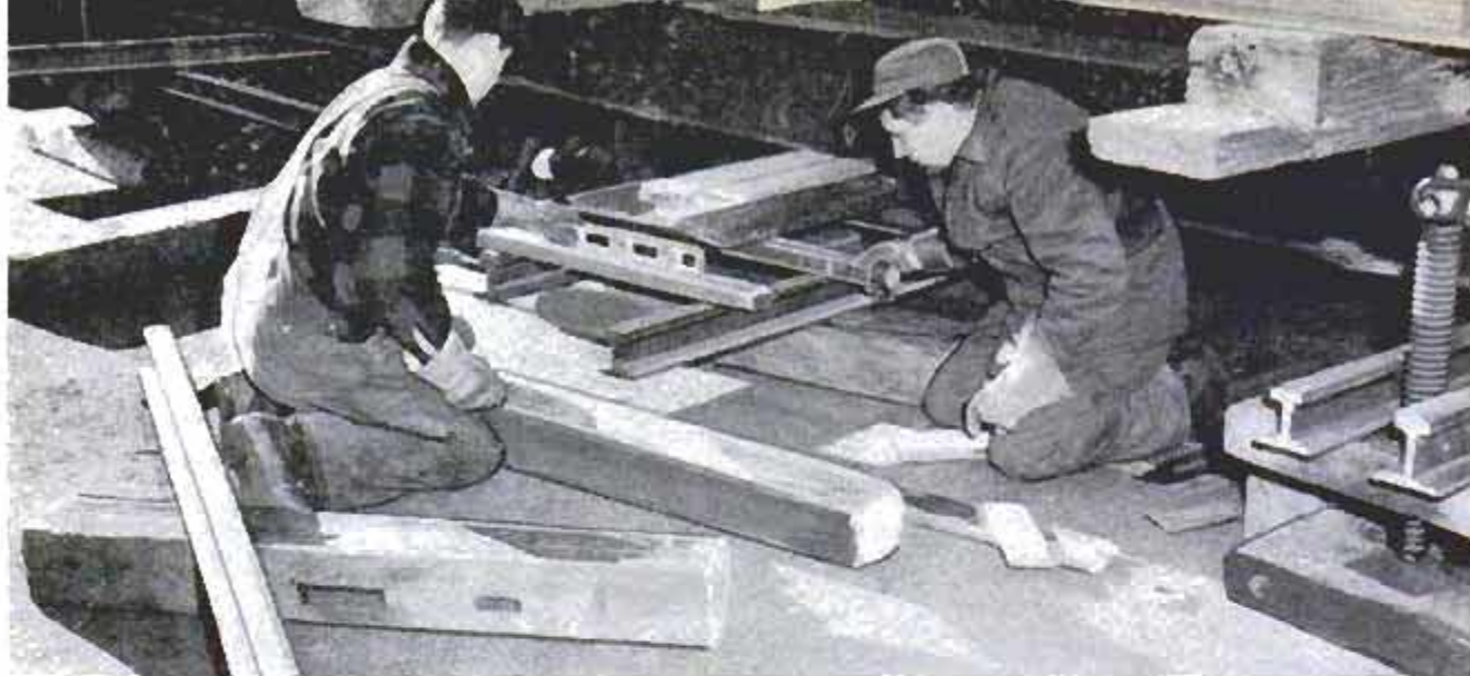
Workmen use level to check tracks on which the hangar rides. Unless kept level, building would splinter
