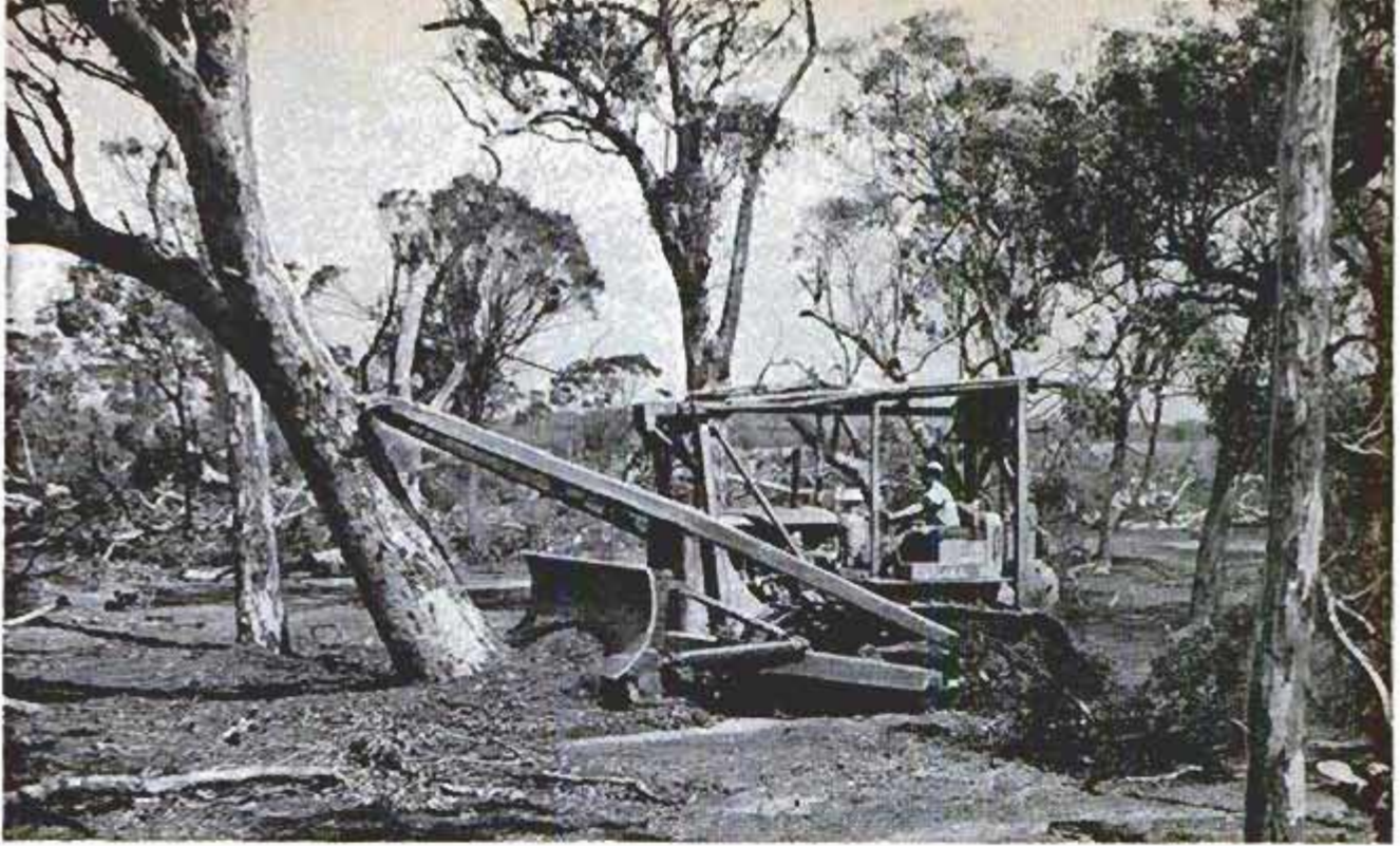
Australia: Mighty mechanical muscles push over a tree to clear the way for a road, opening up new land
