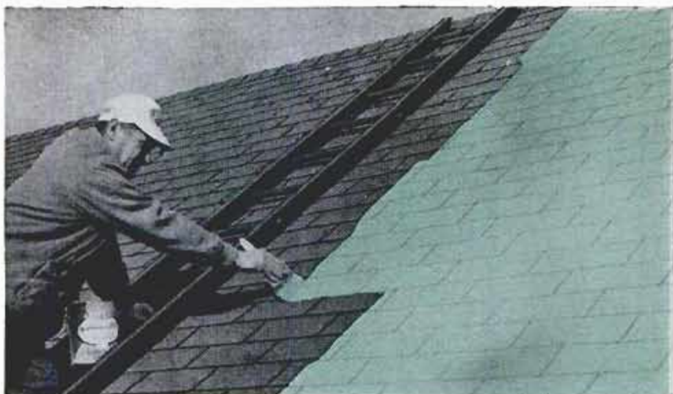
Mr. Tanzillo brushes on a new, metallic green roof, saves cost of shingle job. Sipes Luma-Tint Colored Aluminum Paint is made by James B. Sipe & Co., Pittsburgh, Pa.
