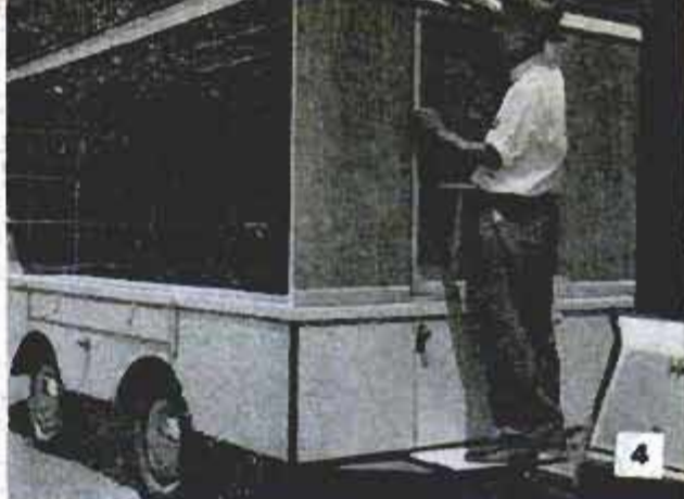
Second step is repeat of preceding operation on wall at opposite end of trailer. Setting up trailer can be a one-man job, but goes quicker with two
