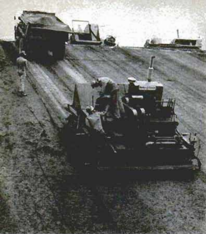
Loaded asphalt truck hangs precariously on the steep slope as it is lowered by cable to the lay-down machine. Spreader lays down a strip 12 feet wide as it moves up dam. Four layers of asphalt were applied
