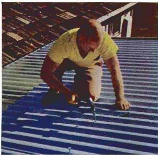
Corrugated Flexboard roofing was easy to nail down. Lighter section nearest house is translucent glass fiber which helps light interior of house as well as the outdoor room. Riley used 12-foot lengths of the Flexboard and 3-foot lengths of skylight paneling
