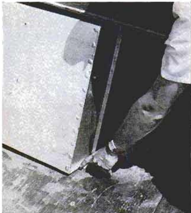
Fig. 6. Fuel-tank leak can be detected by gasoline odor, or stained metal if area of leak is visible
