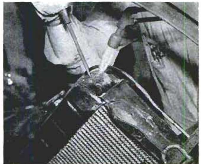
Side brackets are set in place and ends are soldered to upper and lower tanks of radiator. This is the final step in reassembling reconditioned radiator
