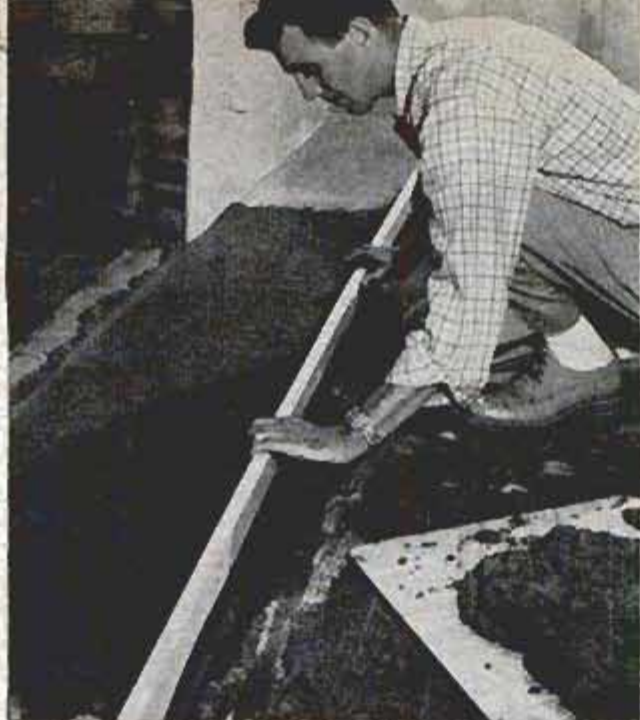
Mortar over brick hearth brings it flush with plywood nailed to floor on both sides of fireplace
