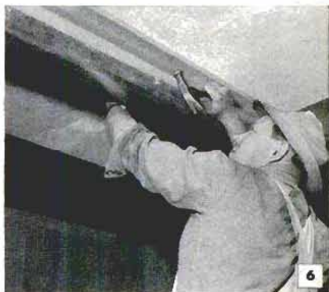
Centered over the horizontal duct, a length of 1-in. stock is nailed to the ceiling to provide a means of supporting the "beam" to be fitted around the duct
