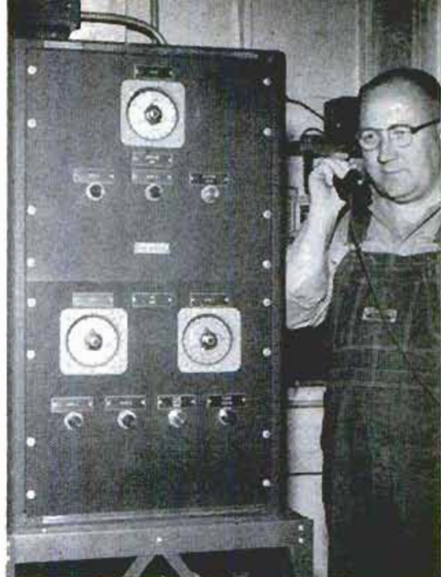
Plant agent telephones dispatcher in Whiting. Line also connects to automatic equipment beside agent
