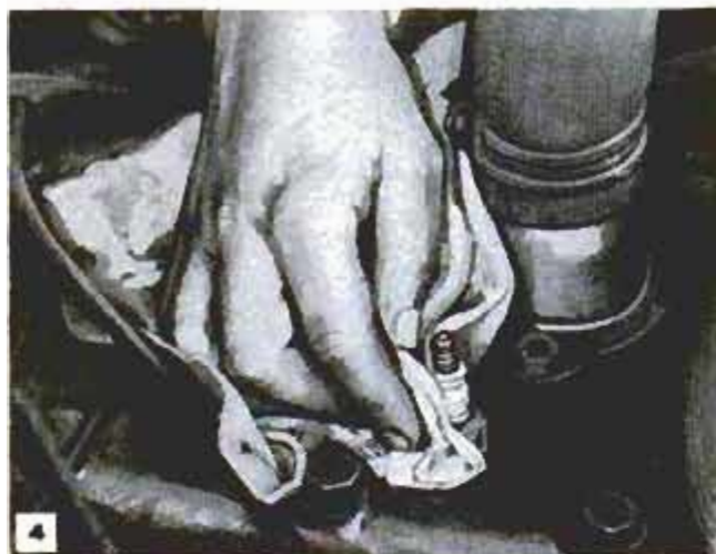
4 After plugs have been loosened, clean dirt from around plugs, so that it does not fall into cylinders
