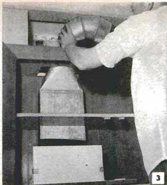
After hood is attached and ductwork run up through cabinet, right-angle elbow is installed in soffit space to route ducting horizontally across ceiling
