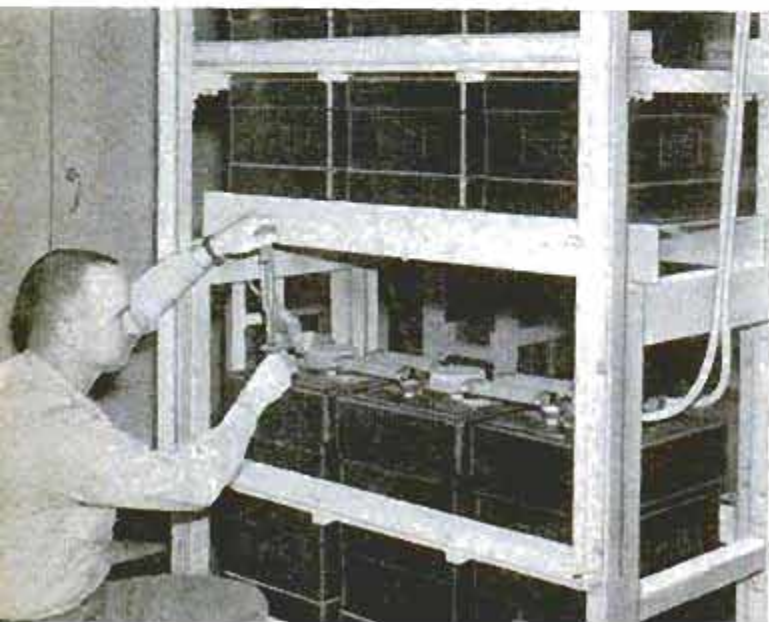
White Alice stations would continue operating if generators failed, using 12-volt storage batteries
