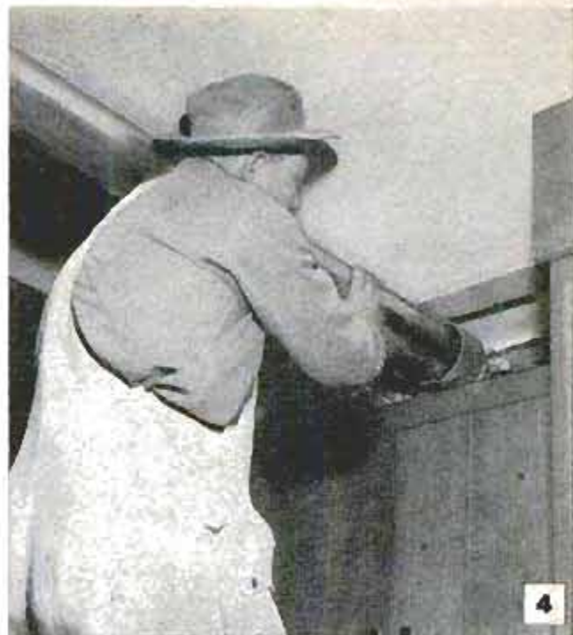
Installation is now complete up to ceiling. Horizontal lengths of ducting now are fitted and run to opening that has been cut through outside wall
