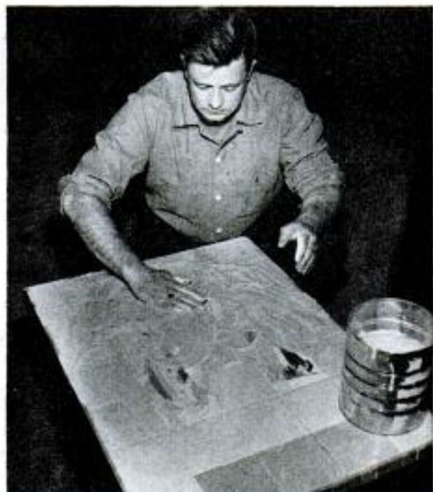
3. Grout is worked into tile joints by moving palm of hand with circular motion over surface of table
