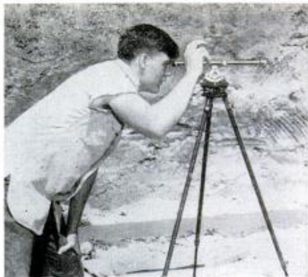
Students in industrial-arts courses started their project by staking out the site for the house
