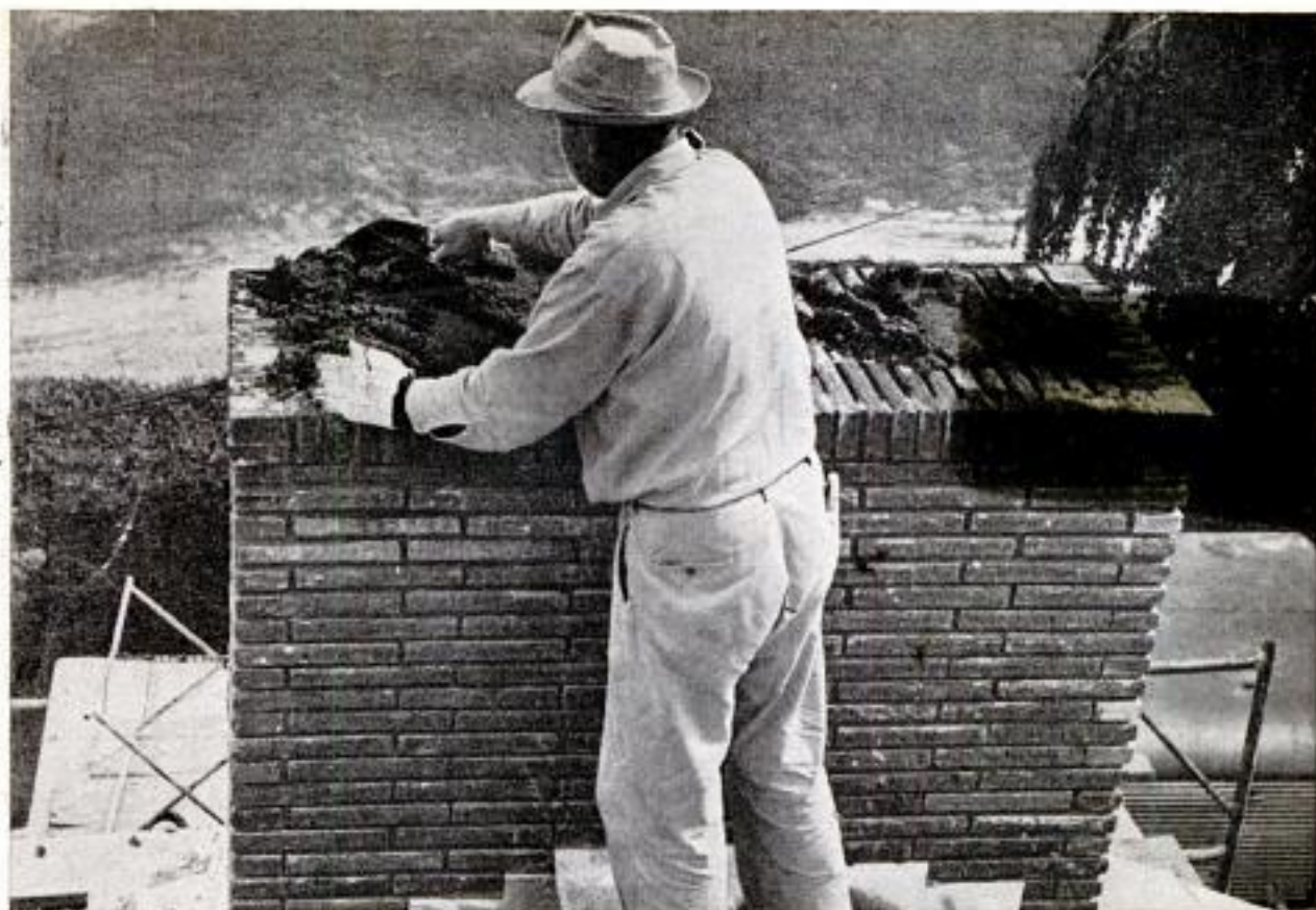
Openings between bricks are filled with a grout made by mixing 1 part portland cement to 3 parts sand
