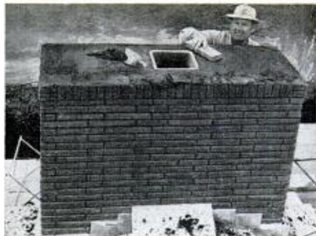
Grout is forced down between bricks with short 2 x 4. Flue can be flush or left projecting a few inches
