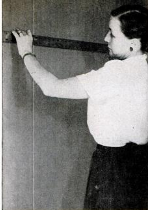
Plumb line is dropped 23 in. from corner. This tests trueness of corner and provides guide for first strip
