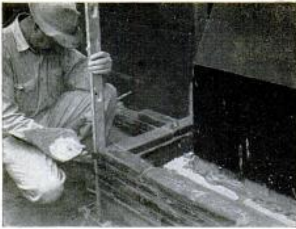
Because of rough texture of Roman brick, side of level is used to check corners
