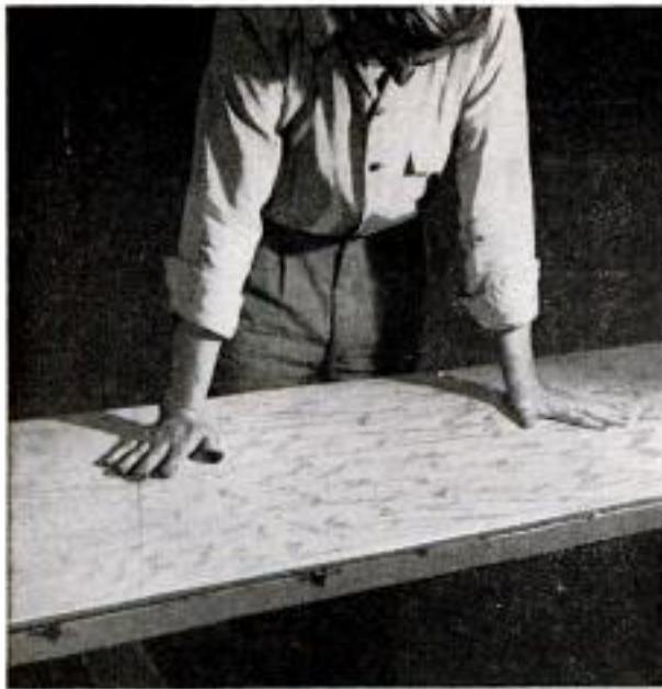
Plywood is pressed firmly into mastic at all points, weights are applied and mastic allowed to dry 24 hr.
