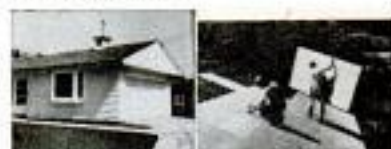
Two-car frame garage amateur can build and getting garage under cover with large sheets of plywood. Both illustrations from the book.
