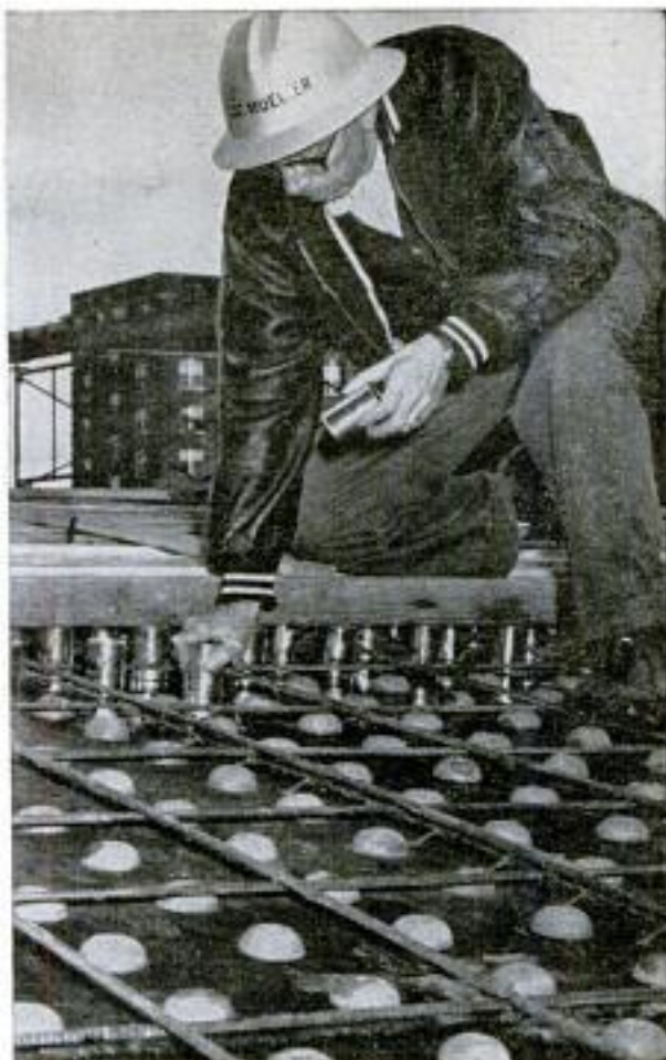
Workman places empty baby-food tins over rubber balls cut in half and nailed to concrete form. Two-by-fours held cans in place while concrete was poured
