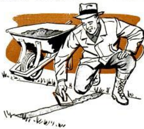
Wooden float then is used to smooth freshly poured concrete. Steel tool is used for final finishing
