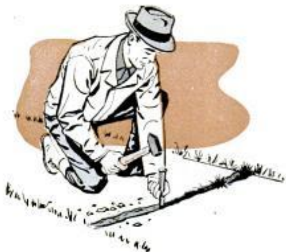
First step in sidewalk repair is to remove old concrete and undercut crack to assure "keying in" repair
