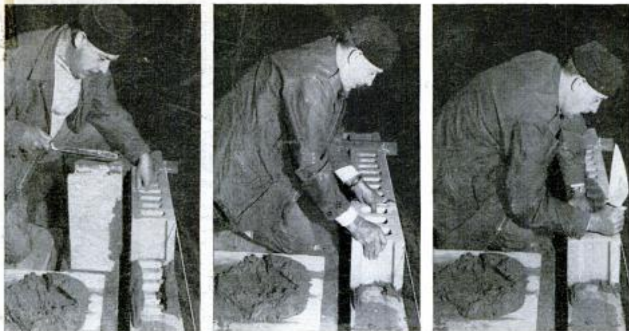
Three steps in fitting block in concrete-block wall are shown above. A ribbon of mortar first is troweled along edges of top of lower block. Also, although not shown, mortar is spread along edges of end of adjacent block. Next, block is lowered into place and tapped into mortar on lower block and adjacent block
