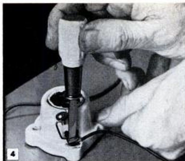
4 Lower end of wire is fastened to screw holding shell in socket. Upper end of wire connects to lead running to strip that is center contact of porcelain socket
