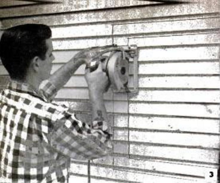
After marking through-the-wall opening on outside, plus the cutting line for the surround casing, a portable saw makes quick work of cutting the opening
