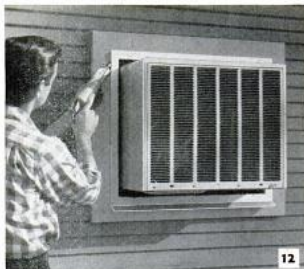
Caulking space between the metal sleeve and surround is filled all around to make it water and air-tight
