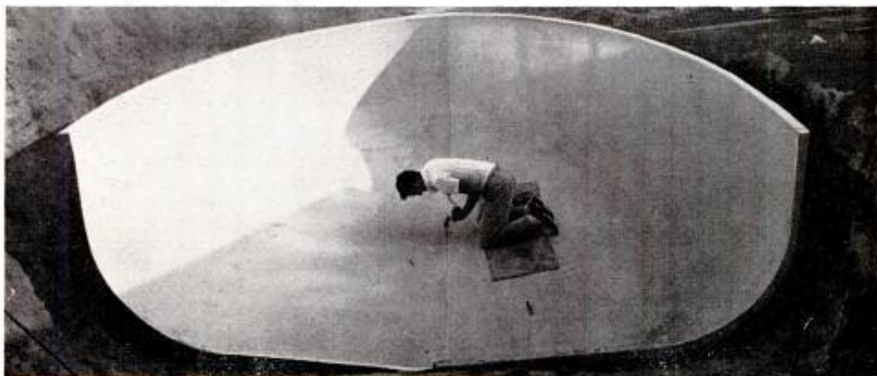
Sections of the glass-fiber pool are joined with screws and self-curing resins. Pool rests in a bed of sand
