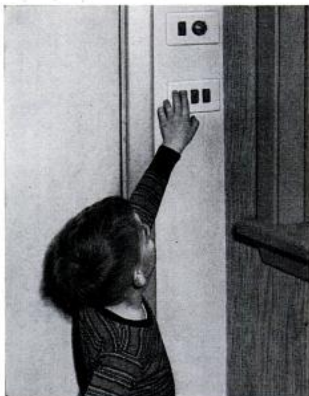
Robert Bear works remote-control-lighting switch. The switches at the top are for lights in other areas
