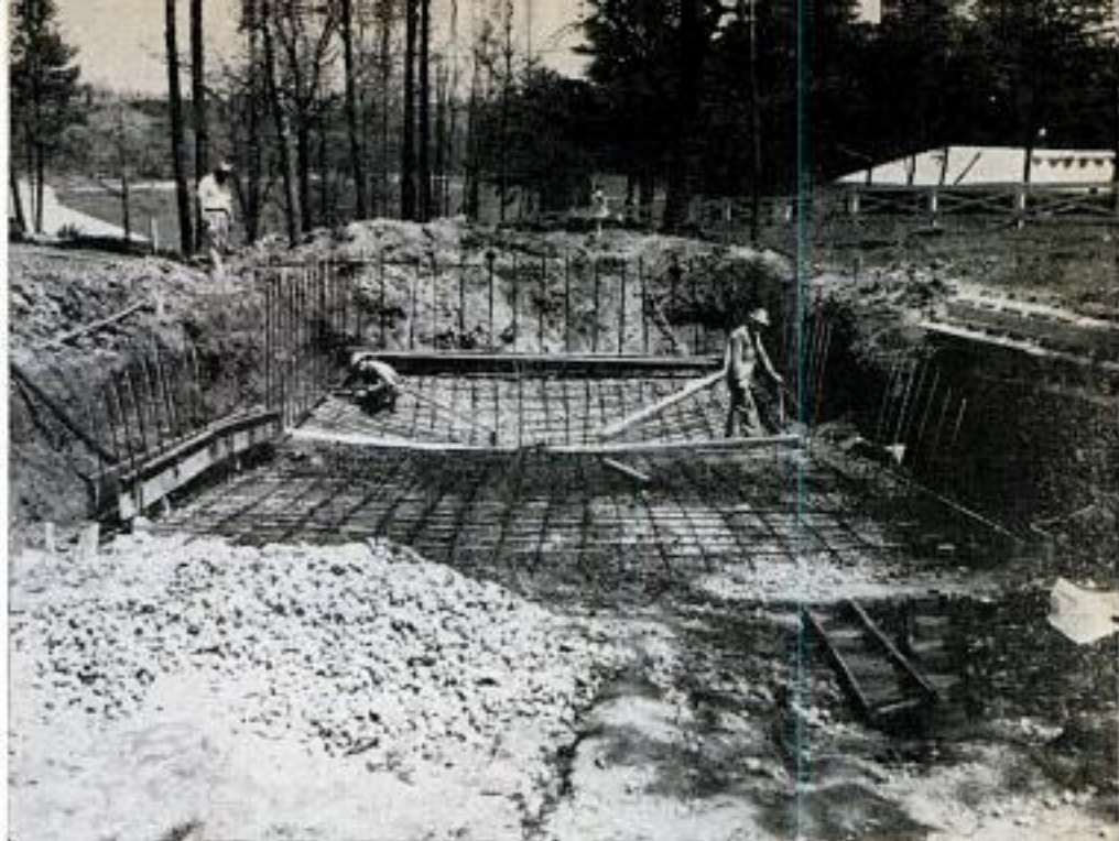
Here are steps in construction of B. F. Aldredge pool. It is a concrete-block, do-it-yourself package. Above, floor is poured concrete, reinforced
