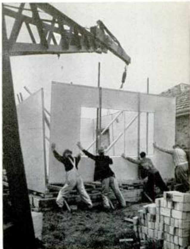
With the conventional foundation and floor joists in position, plaster walls are installed by crane
