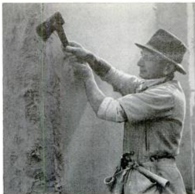
Plaster and sisal fibers at joined corners of the house are trimmed to allow placing of brick veneer
