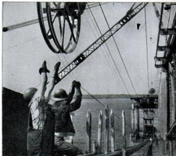
As wheel travels along, wire is payed out. Bottom wire is dead and is pulled down to be part of cable
