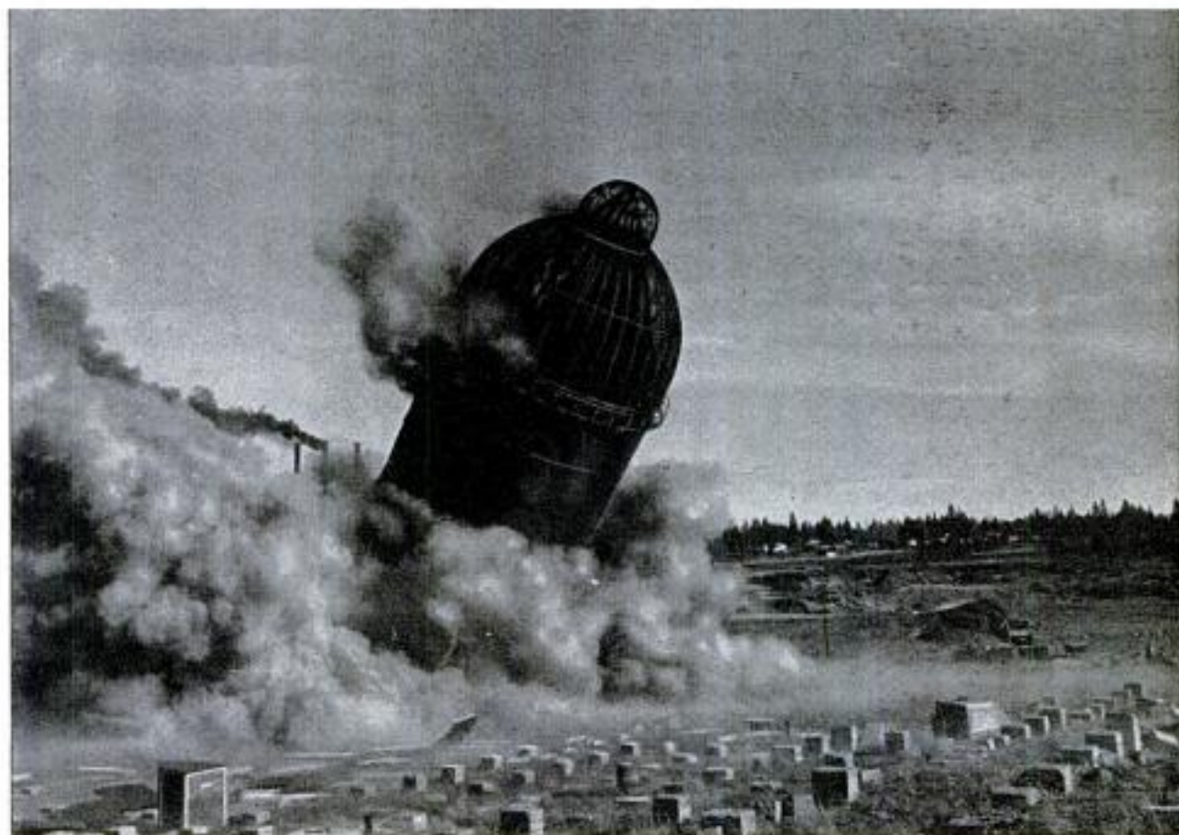
Ancient scrap burner weighing 835 tons came thundering down, much as a tree falls in the direction controlled by woodsman's ax. When dust cleared, demolished burner was lying exactly along predicted line
