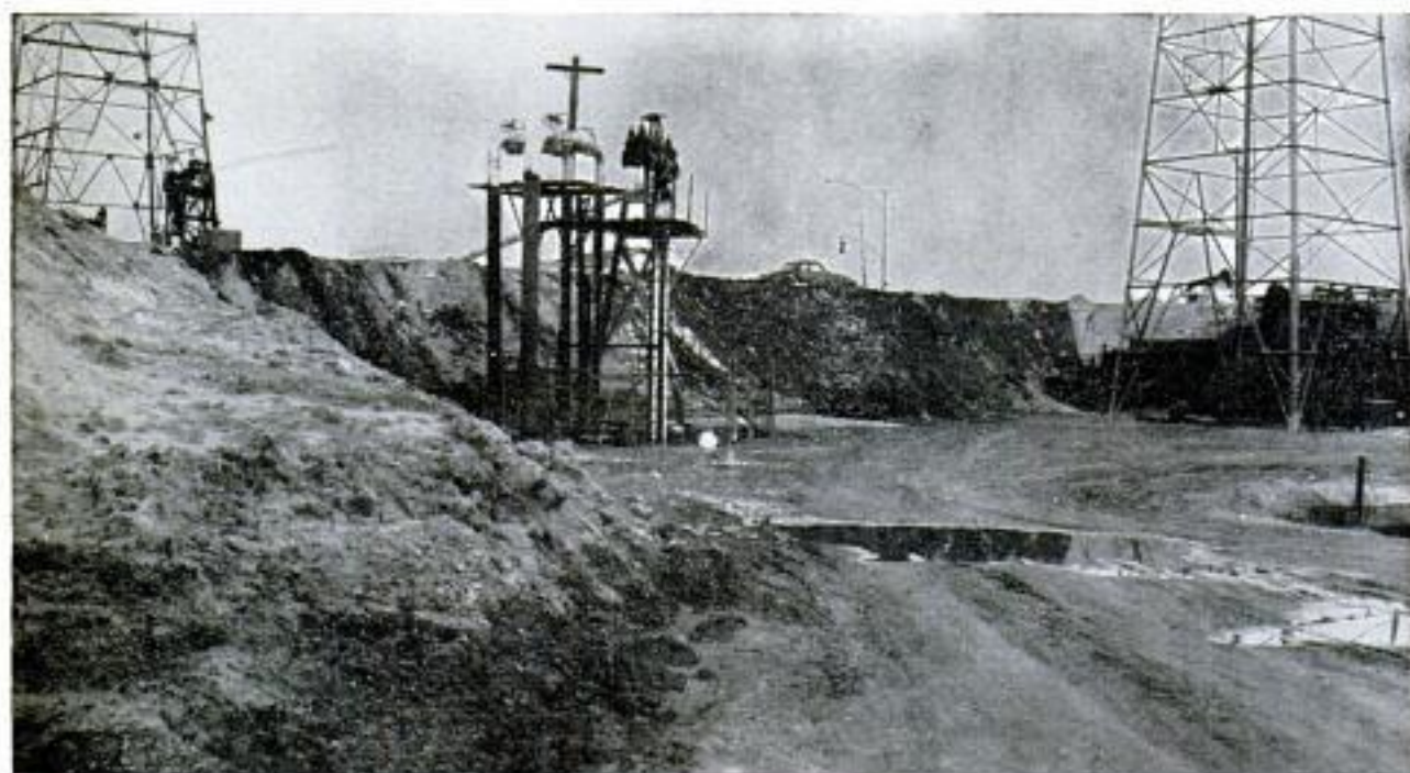
Well head, center rear, will be at ground level when earth-fill operations upgrading the area are finished
