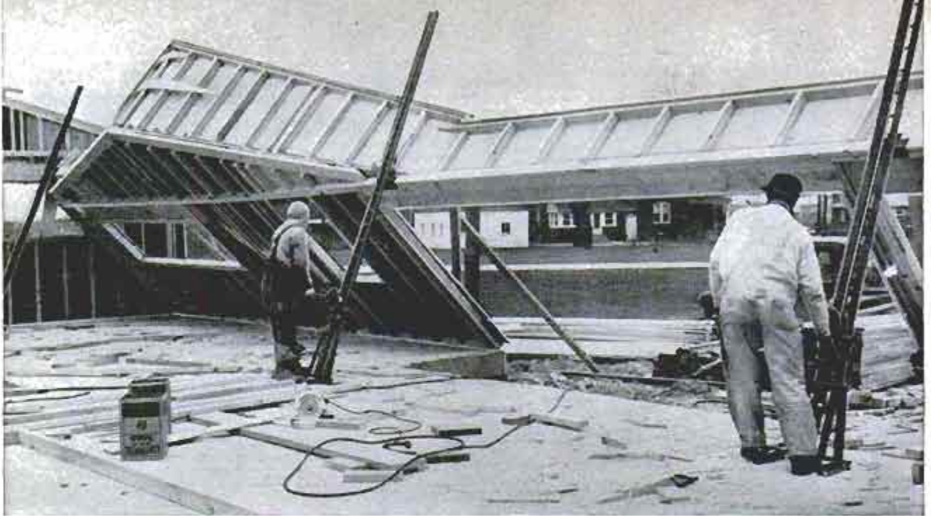
Workmen crank entire wall section of residence into position. Safety dog prevents falling if cable breaks
