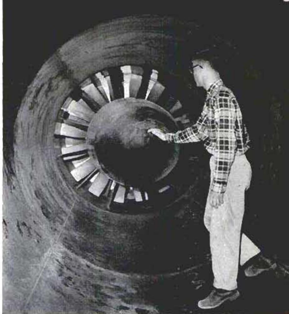
Each intake fan is capable of pushing 220,000 cubic feet of air per minute into the tunnel. Blast cools hard-working diesels
