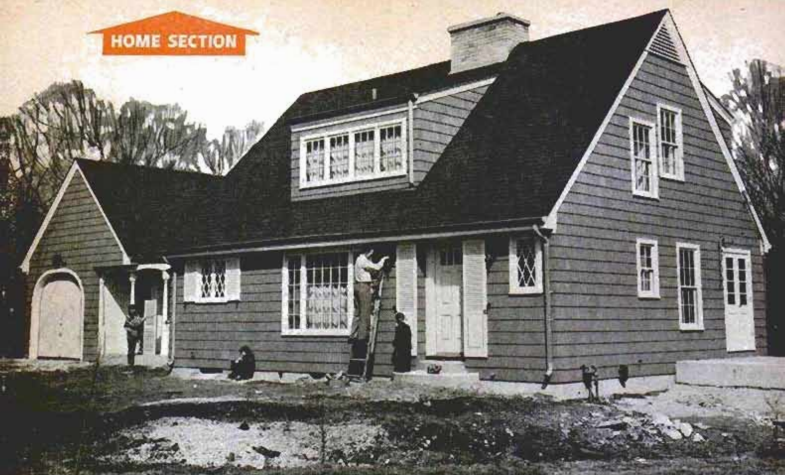
The Murphys at work on their new home—Frank attaches light fixture and Evelyn is busy fitting shutters
