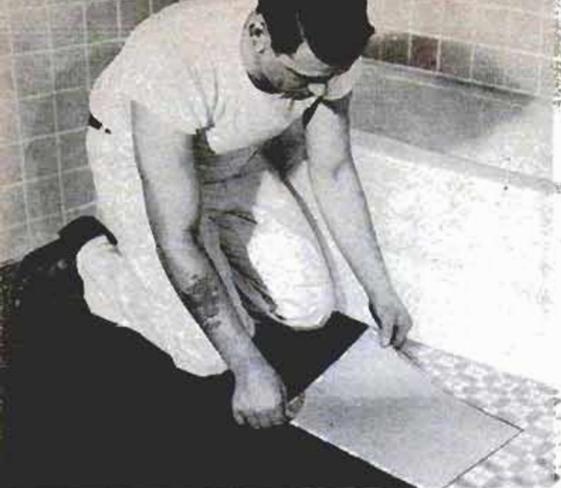
After sheets of tile are aligned they are forced into adhesive and leveled with tile-setter's beating block
