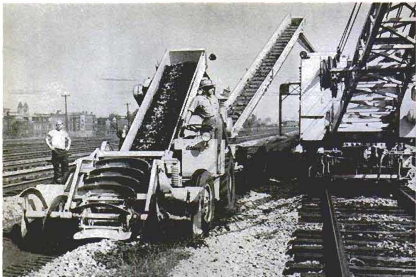
Scrapers on endless track shovel rock onto conveyor. After screening, cleaned rock is dumped into boxcar
