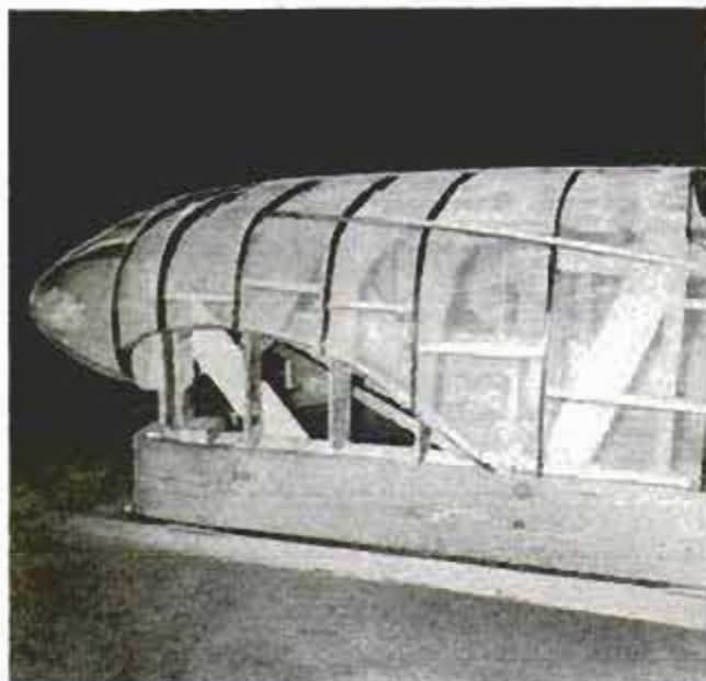
Wood templates covered with screen were assembled like this to form a frame for the plaster mockup
