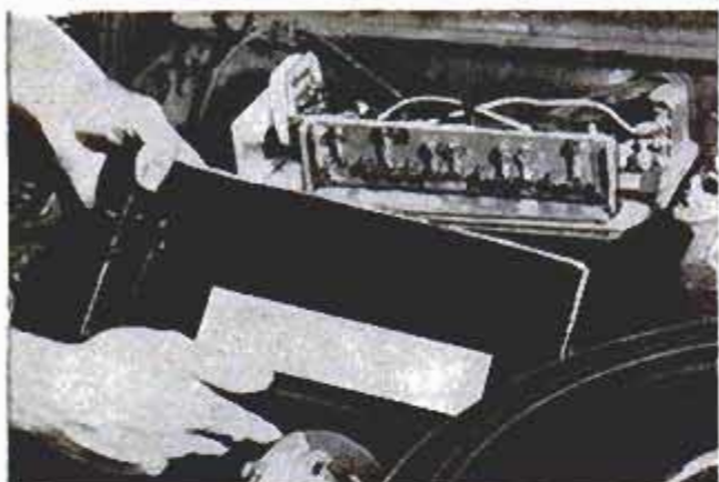
Convenient fuse box has its circuits labeled in lid
