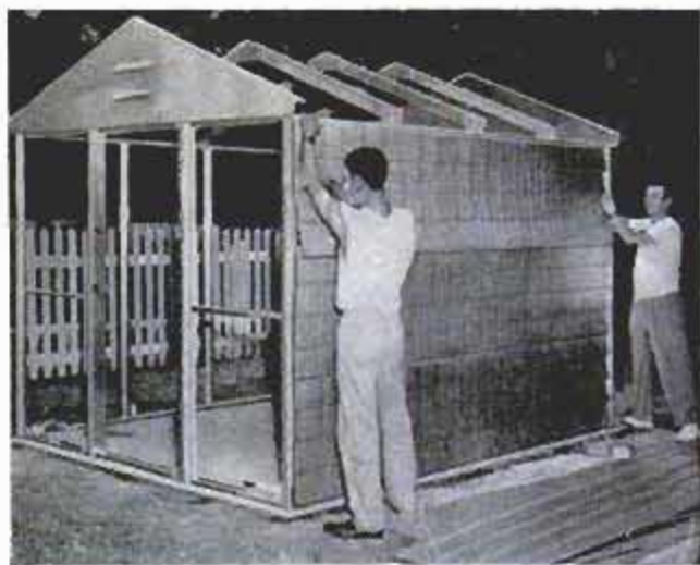
Side of room is made up of three sheets of aluminum. The roof rafters are preassembled to minimize work
