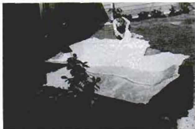
After hole has been excavated and wet soil smoothed with broom, cut glass-fiber cloth to fit in pond
