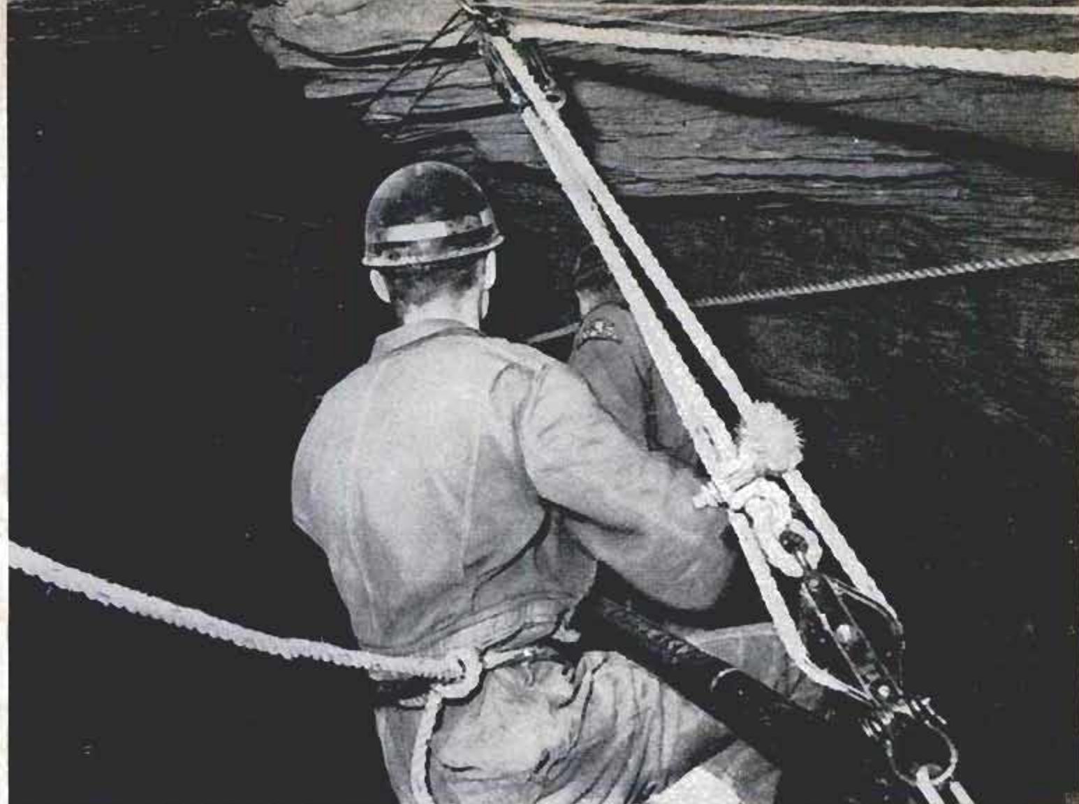
Cables fastened to the top rung of the pipe bridge hold it in position as the explorers jockey it forward
