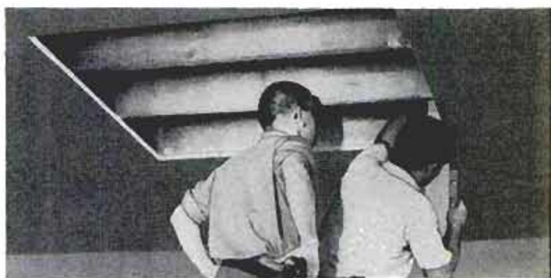
Above, fan opening is cut through garage ceiling, leaving joists intact, after which fan-supporting framework is suspended under opening as below. Be sure framework is level so fan is supported solidly to assure that fan and motor will operate quietly
