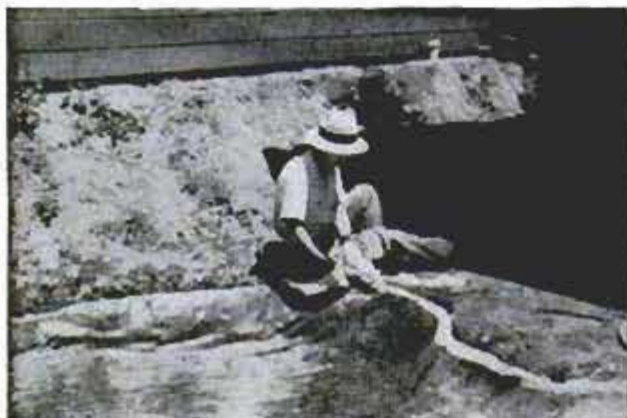
Trim dried cloth with tin snips, paint edge with resin to eliminate sharp edges. Patch all holes
