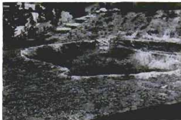
Use paintbrush and saturate cloth with resin. Patch holes with cloth and resin, allow to dry completely
