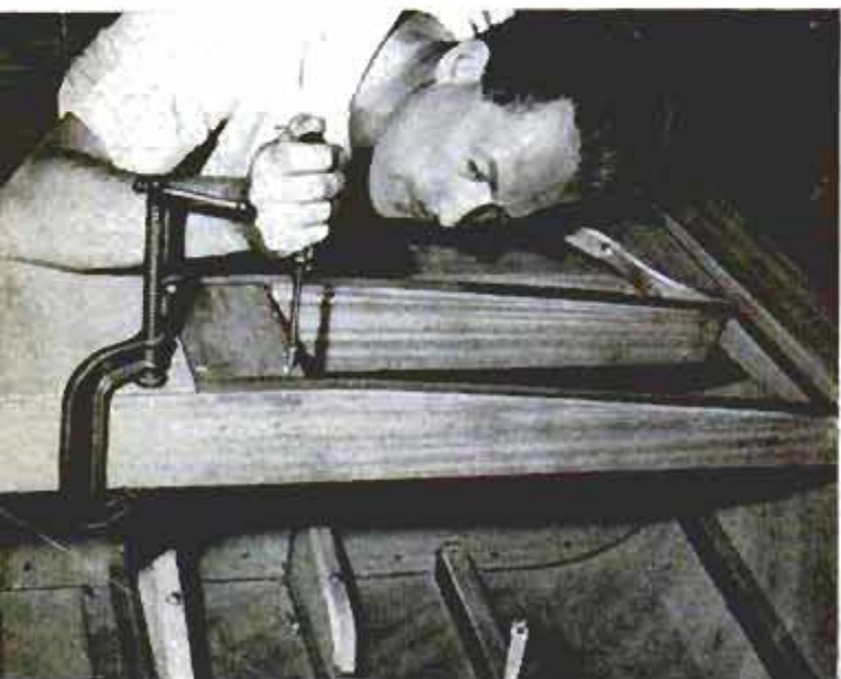
5. Below, removable rear deck is assembled on hull to assure good fit. Marine glue is used in all joints
