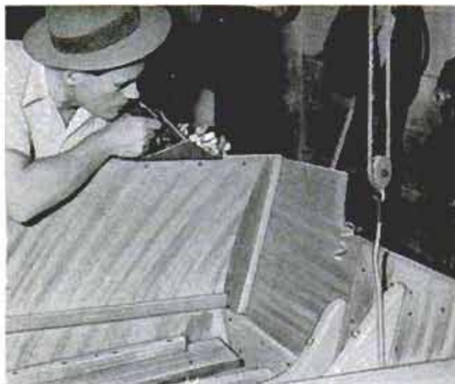
4. Before installing cap rails, top edge of hull is planed to be flush with top edge of gunwale strips
