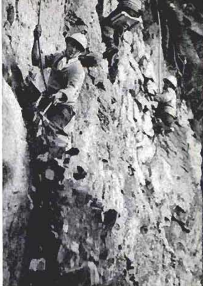
By knocking away these loose rocks and debris, the workmen minimize number of dangerous landslides
