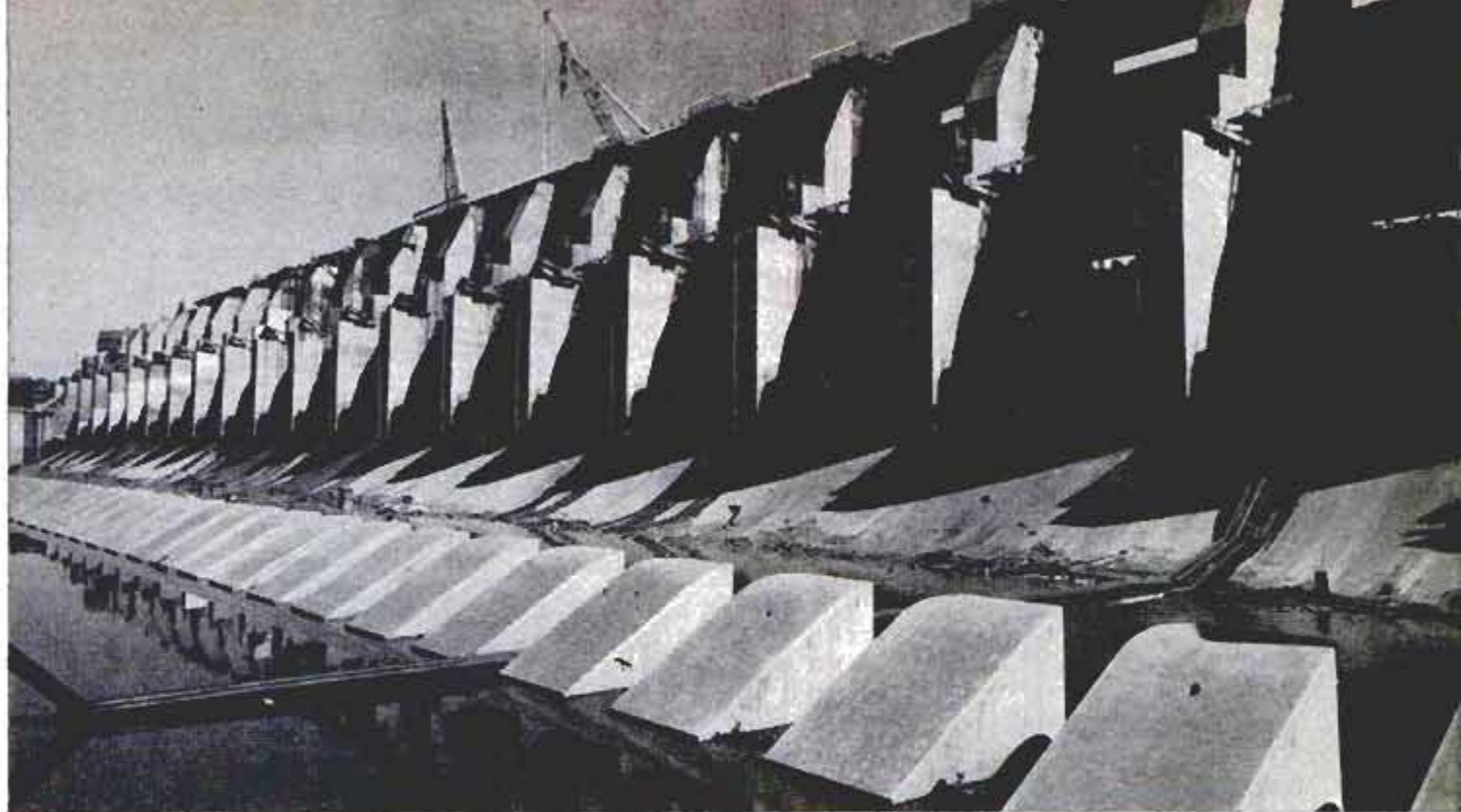
Spillway of The Dalles Dam nears completion. Reservoir will back up 25 miles, cover 11,000 acres with water
