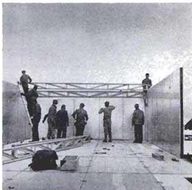
By slipping and clipping pieces together Seabees erected one 24 by 48-foot building per day . . .
