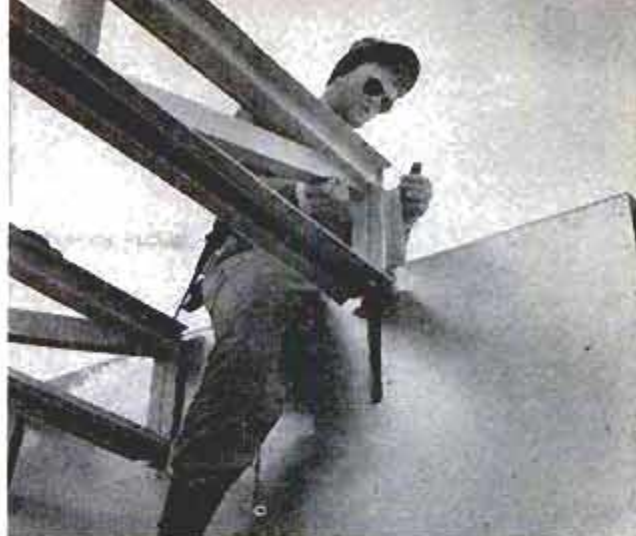
Ceiling beams fit into slots in side walls of huts and help to make the entire structure rigid . . .
