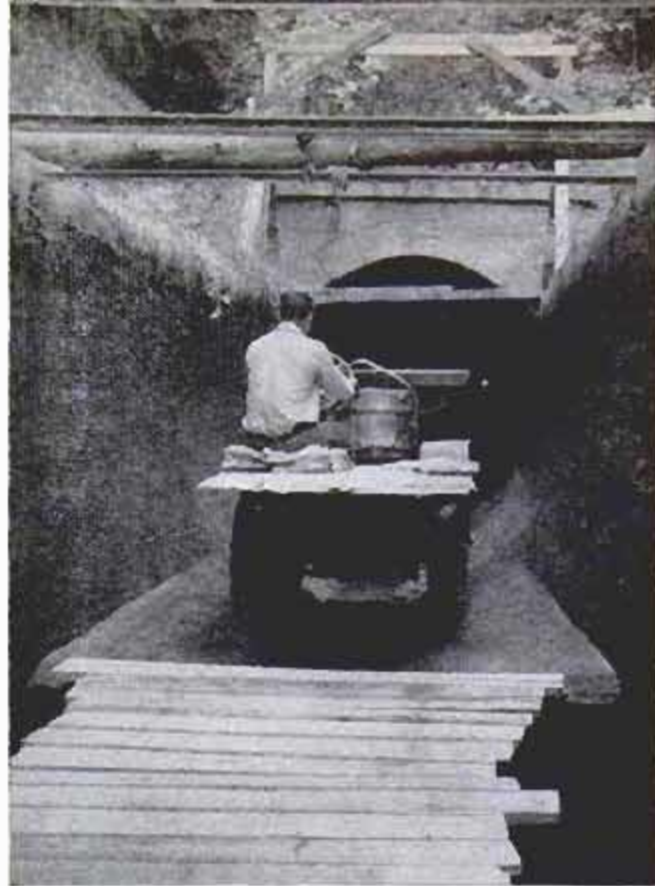
Planks are laid over opening of huge sump valves to allow car to pass. Valves release water in emergency
