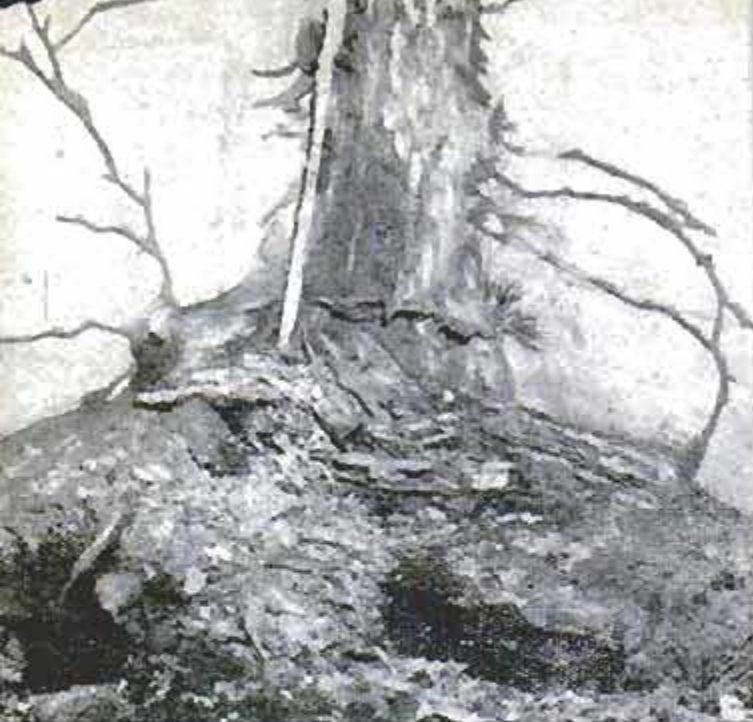
Shelter tunnels built by a termite colony on the inside of basement wall in order to reach wood above
