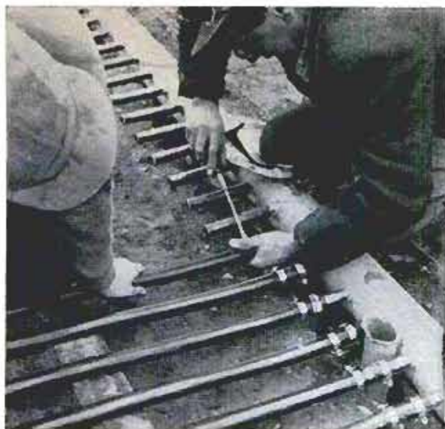
Plastic tubing to carry refrigerant is connected to the supply pipe in Wilmington, Del., playground rink
