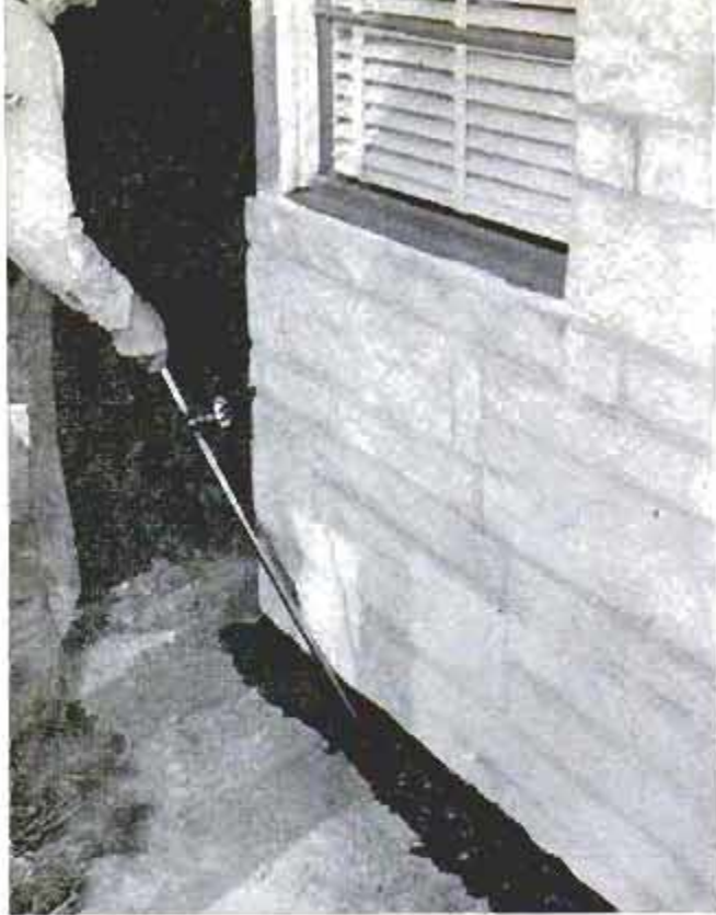
After trench has been filled, fresh earth is thoroughly saturated with a suitable chemical solution
