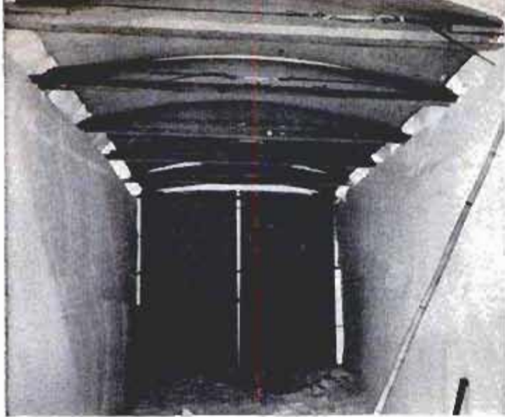
Removable arched plywood forms are set in place over trench, two feet down. Snow will be blown on top
