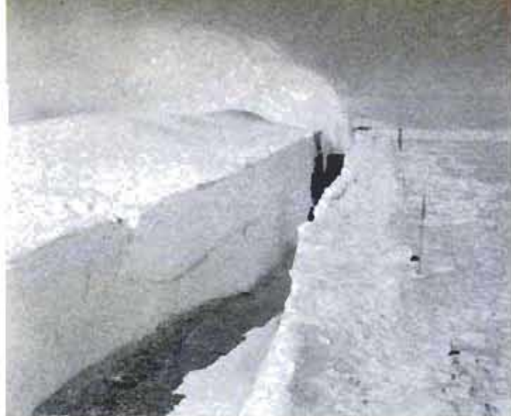
Digger cuts a trench eight feet wide and three to five feet deep at each pass, blows snow out the top
