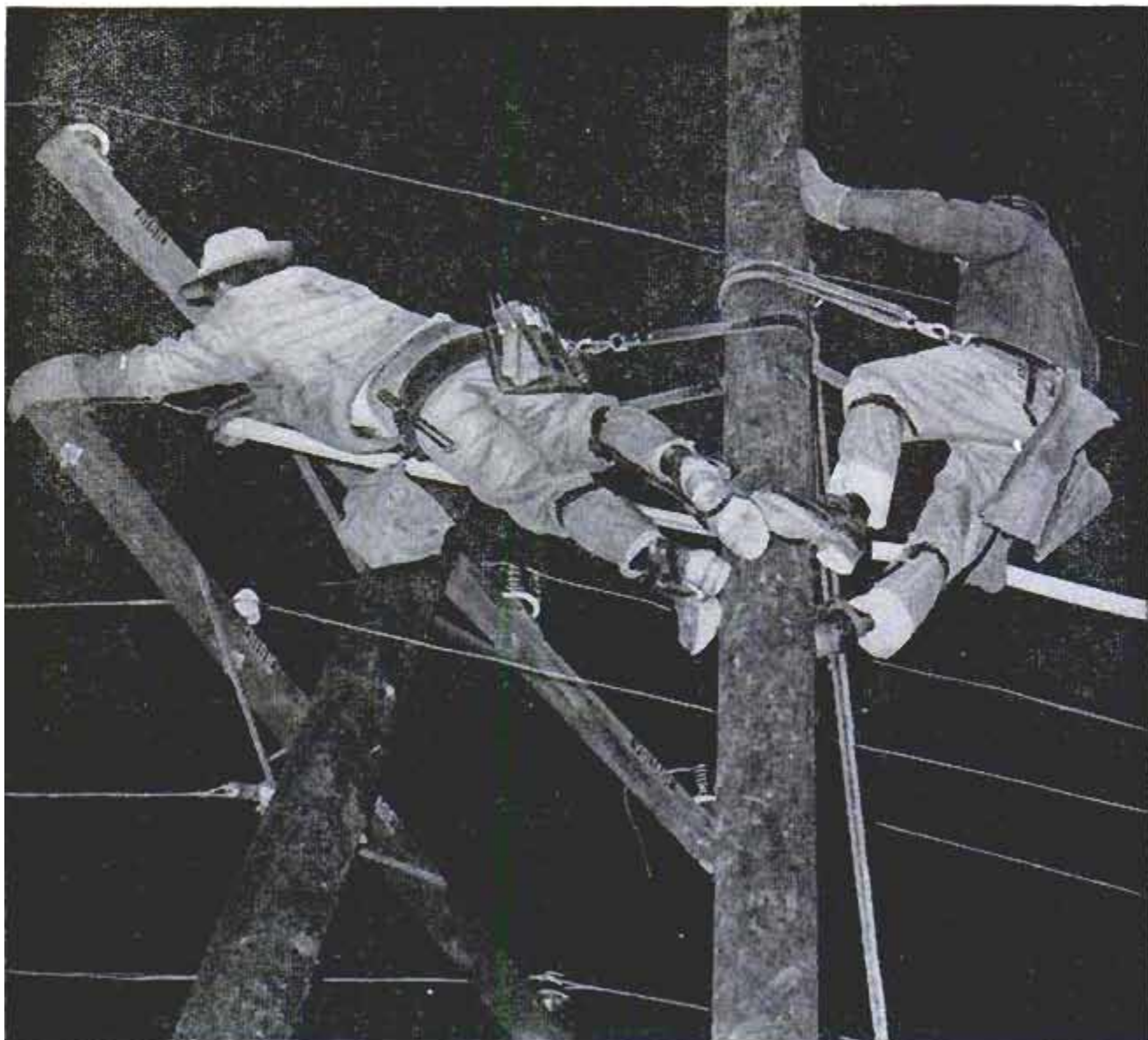
Lineman leans 'way over to slide rubber "snake" over wire. Voltage here is 4000 volts phase-to-phase
