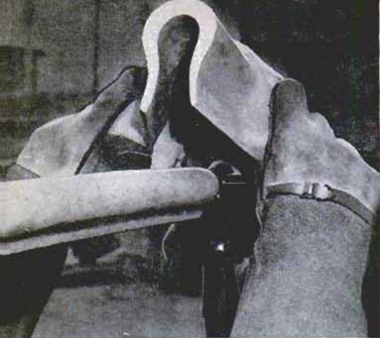
Rubber hood is placed over an insulator to protect workers on power line. Rubber "snake" covers wire
