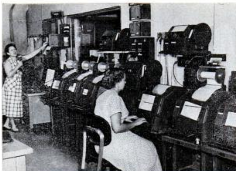
Teletypes line wall of Communications Center. Slave units of these machines are installed in police, fire stations of Miami and suburbs
