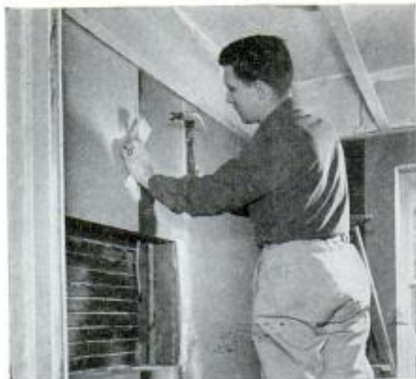
Molding is tapped in place by using wooden block to cushion hammer blows. Adhesive anchors molding
