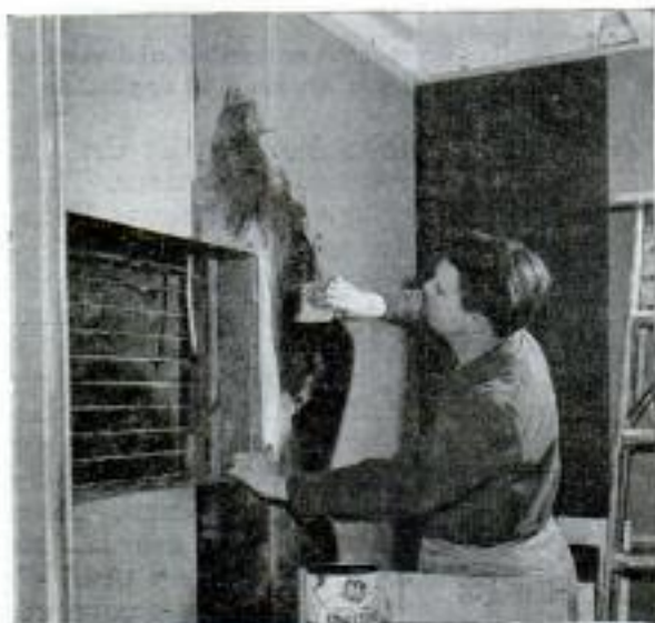
After next piece of laminate has been cut to size, adhesive is spread on wall surface and on laminate
