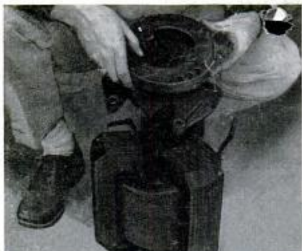
3. Pole transformer is removed from its oil-filled tank and distribution ring and wire leads discarded
