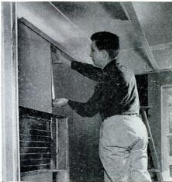
Divider molding is added to edge of laminate already in place. Molding is cut short to clear medicine cabinet
