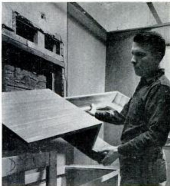
Plywood top for lavatory is assembled and checked for fit before the plastic laminate is applied to it
