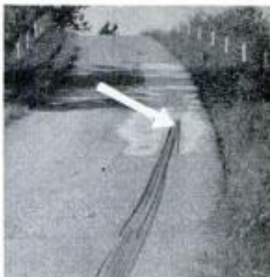
3 Car can climb no higher than point of arrow even though its left wheel is on clear pavement
