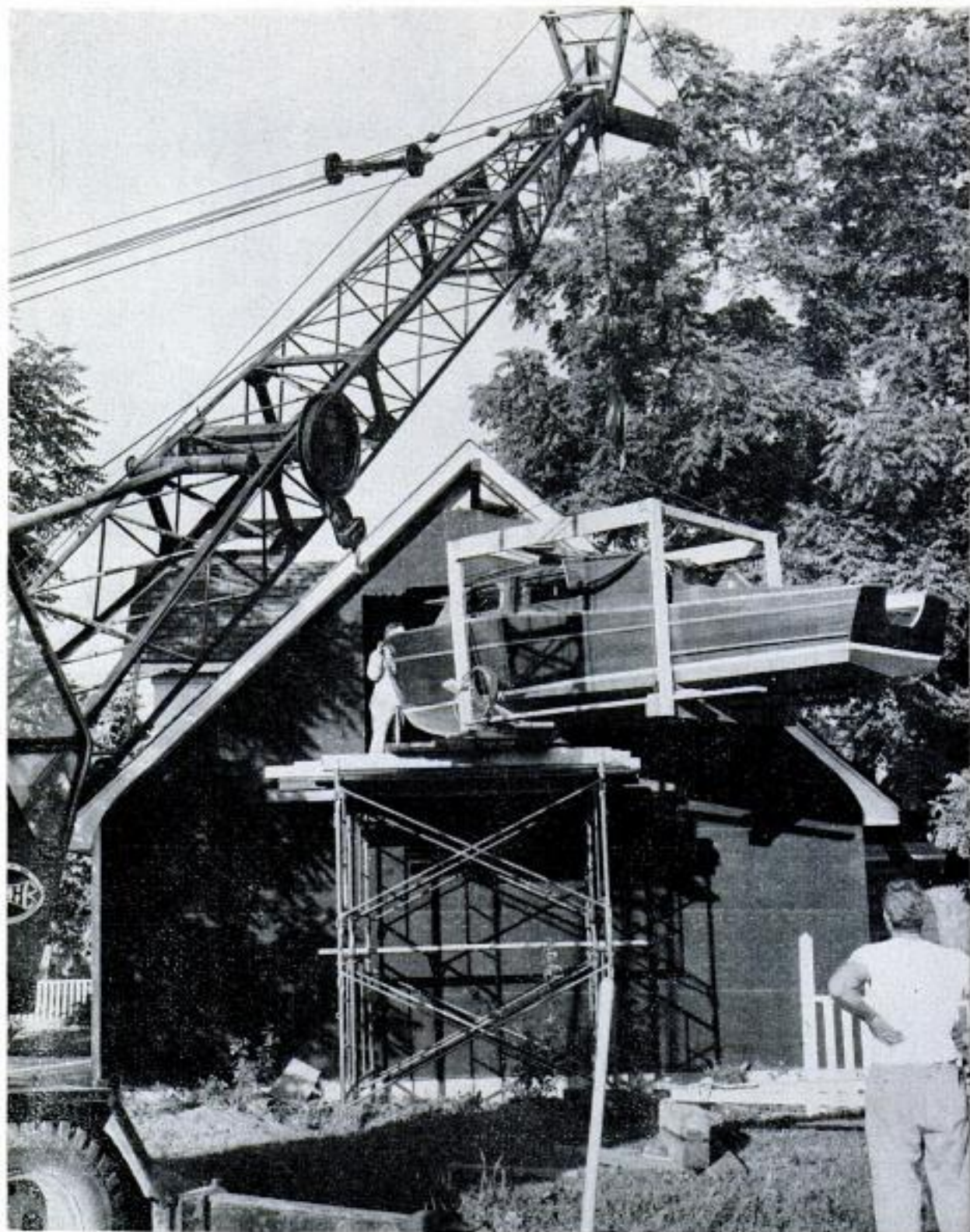
Boat suspended from crane swings off launching platform. Hole was cut in side of house to get boat out
