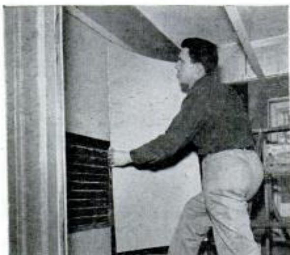
After adhesive loses tacky feeling, panel is slipped in place. Tap corners with block for good adhesion
