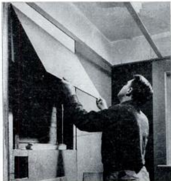
Hardboard or 1/4-in. plywood panels nailed to studs provide smooth surface for application of laminate
