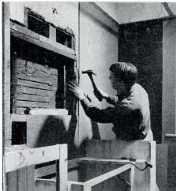
Lavatory framing, cutout for medicine cabinet and part of hardboard underlayment are shown above
