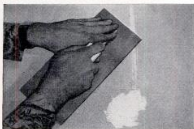
3. Using the edge of the trowel, slice down across the crack to remove excess material. Allow 8 hr. to cure
