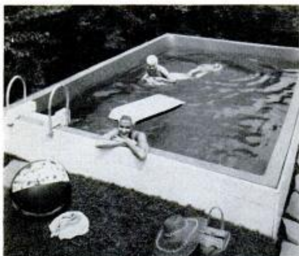
Plastic pool in a small size can be built for less than $500. Liner is fastened inside a wooden frame
