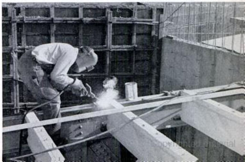
Precast concrete joists 20 feet long support the floors of the lodge. Reinforcing bars in the concrete are welded to the steel roof trusses
