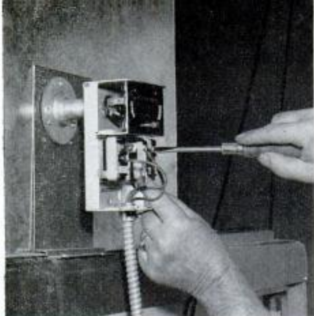
Combination limit control and blower control is located in warm-air plenum as shown in photo above. Below, an automatic humidifier installed in the plenum maintains the correct humidity in your home
