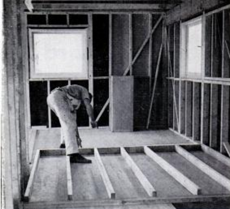
Partition walls with single top and bottom plates are assembled on deck, then tipped up into place
