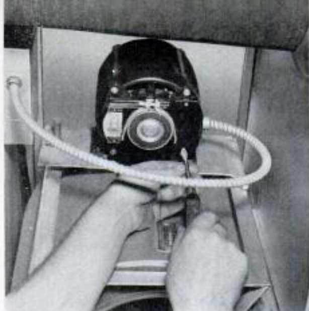
Above, use flexible conduit to the blower motor as it rests on flexible mountings which would fracture rigid conduit. Below, if the furnace is oil fired, an oil filter should be installed in the oil line
