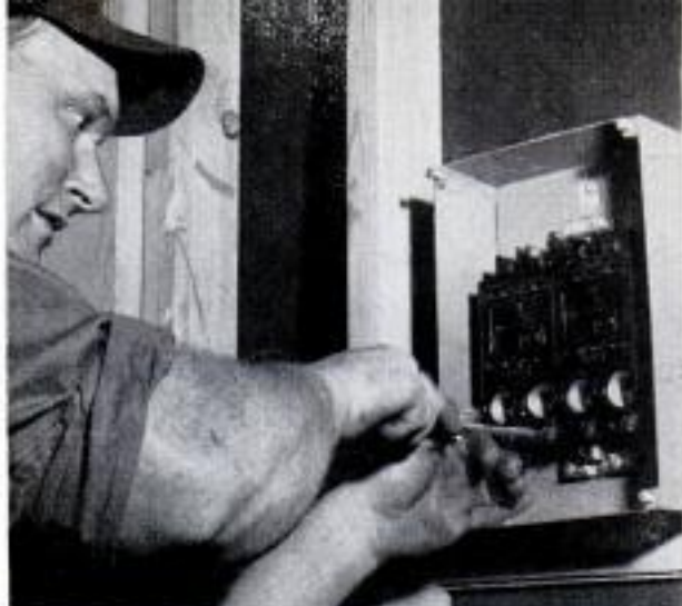
Fuse box to handle all circuits is a four-fuse service located in entry closet right behind meter
