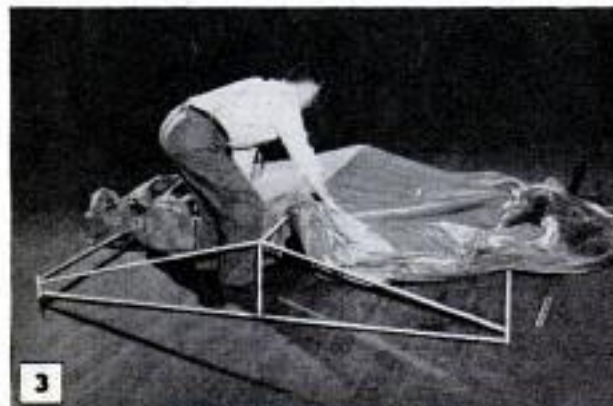
3 Above, second step in setting up is placing canvas roof and screen sides over frame. Below, setting corner posts after roof and sides are in place
