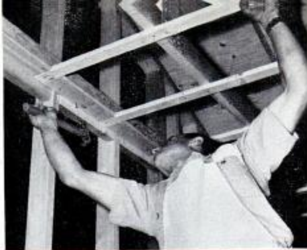
Furring strips nailed to roof trusses support fasteners that clinch big ceiling panels from behind
