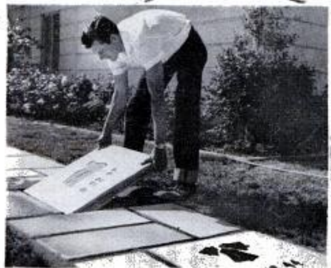
The 2-ft.-sq. block being set in place in photo at left weighs about 90 lb. Smaller rectangular blocks are easier to handle. Cutout designs and impressions are made in concrete as on following page
