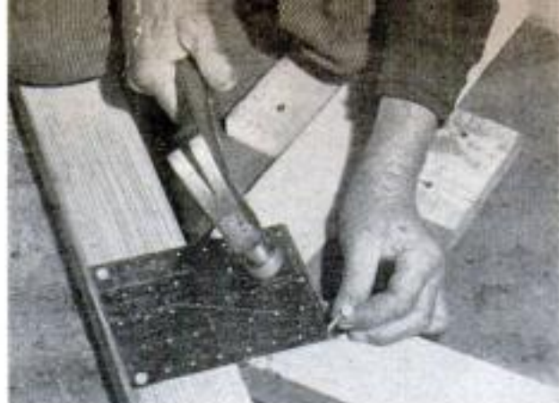
Sides of H-brace are nailed to 2 x 4 truss members with barbed asbestos-shingle nails, as above
