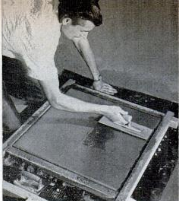
After cutouts are set in place, they should be troweled over to set them flush with concrete surface
