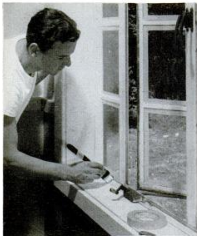
Regular sash brush makes window painting go fast. Masking tape may be used to keep paint off glass
